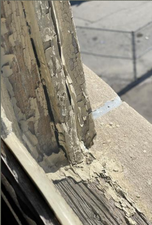
Existing window deterioration
