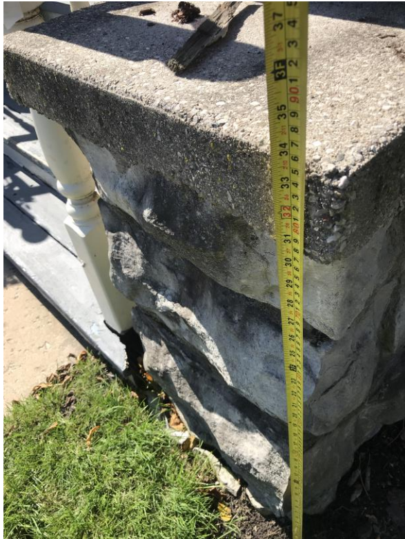
Wing walls measure 32 inches tall by 22 inches wide by 52 inches deep (front to back) They will remain.
