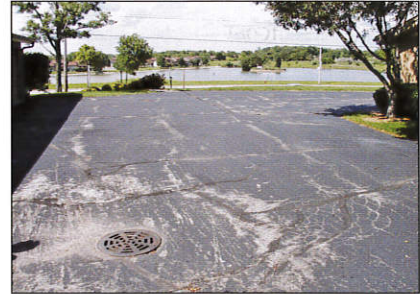
Light gray patches of asphalt show where sealcoat has been worn from the pavement. Applicators recommend reapplication of sealcoat from every 1 to 5 years. 1
