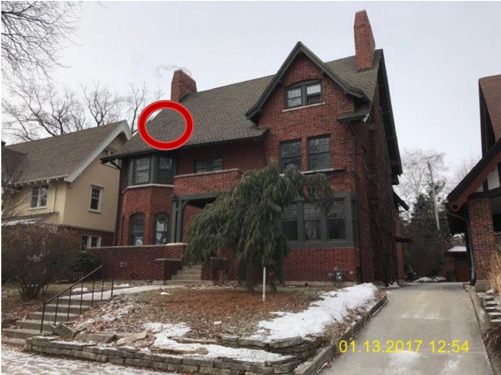
Current conditions. Patch will be made in gable roof at shown location and a new rubber membrane roof will be installed on the porch roof (center front).
