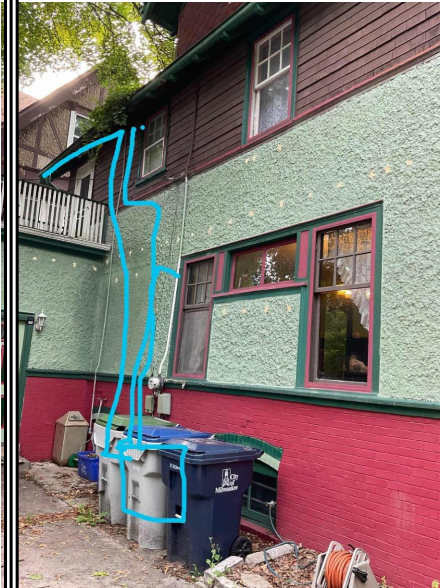
Location of AC at rear of property
