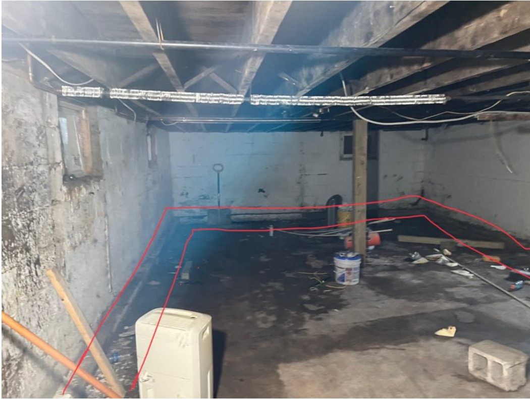
Install 100' of drain tile along 3 walls, including a Bucket well and sump pump with a 2" pvc pipe
