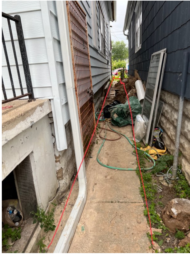
Replace 60' X 3' side wall (this most include any stairway, window or curbs
