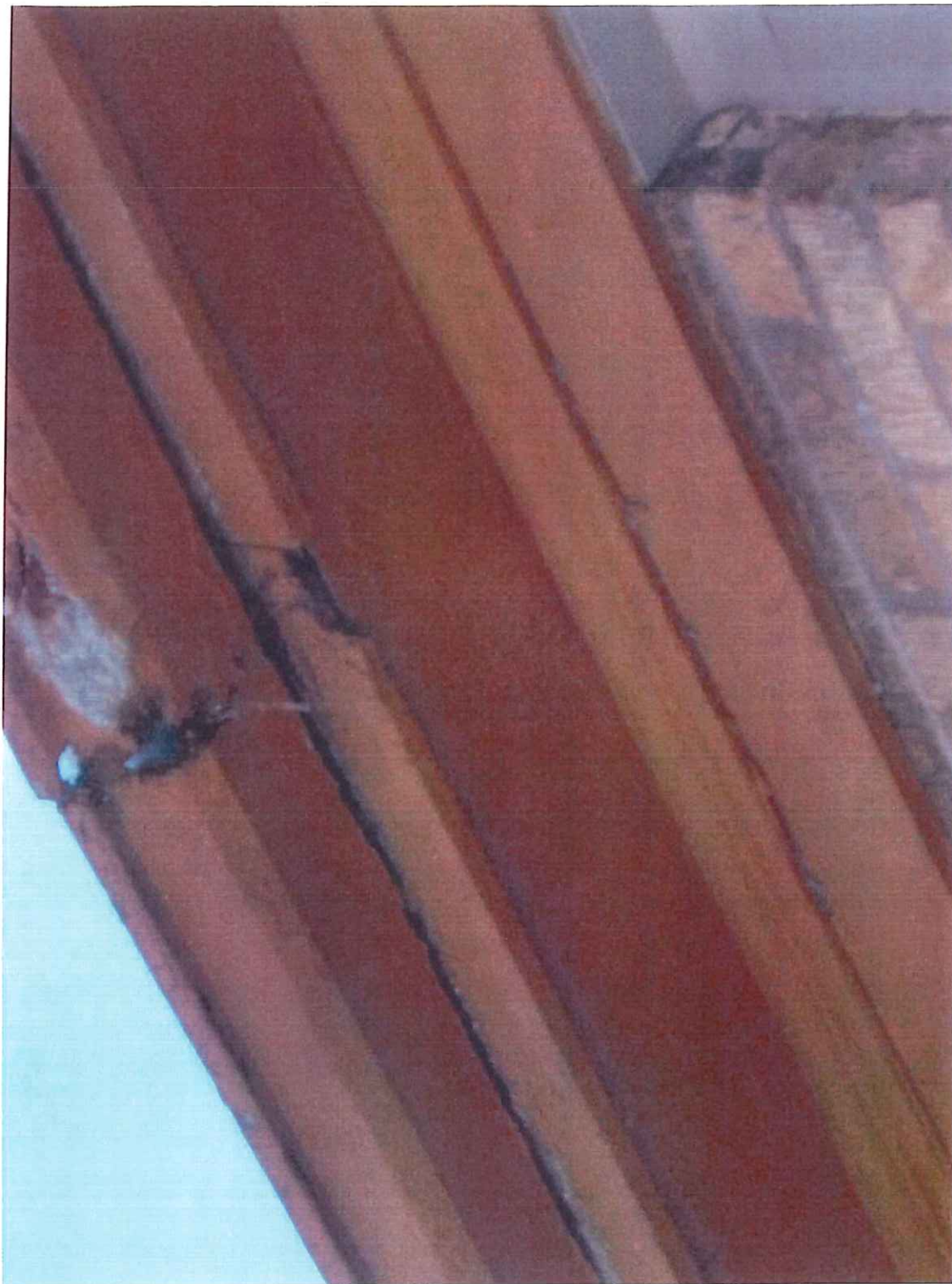
3-15-2023 3624 N 40TH ST JCR VIOLATION # 2
