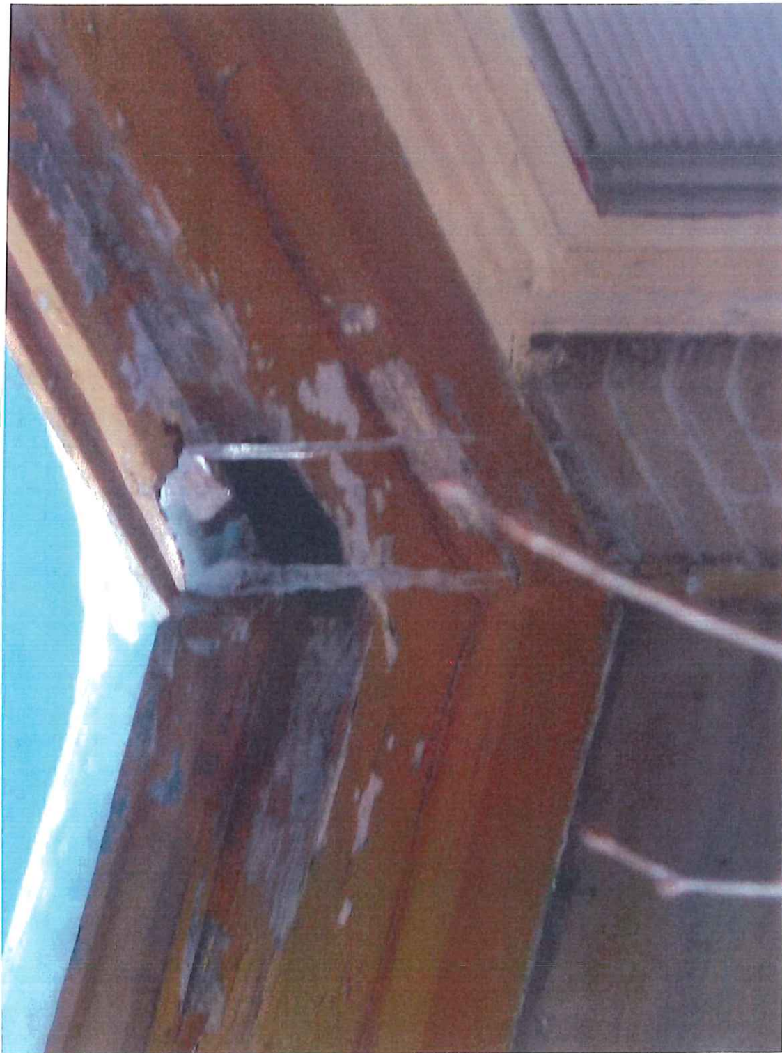
3-15-2023 3624 N 40TH ST JCR VIOLATION # 2
