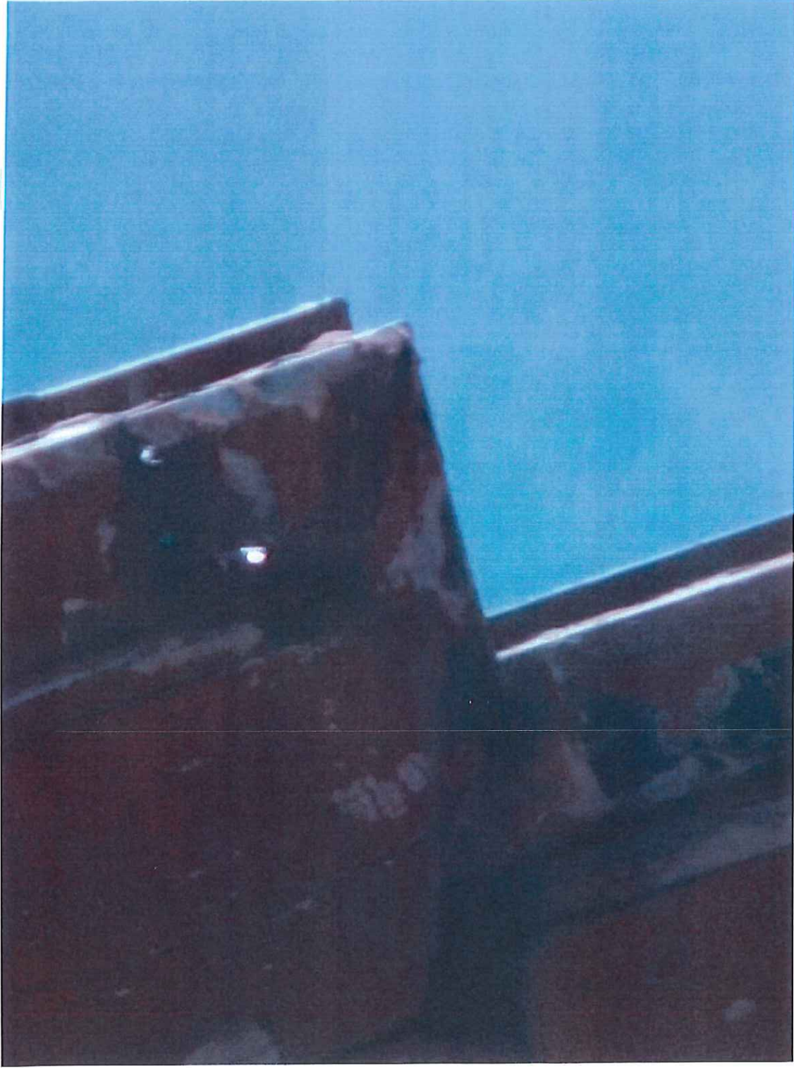
3-15-2023 3624 N 40TH ST JCR VIOLATION # 2 & 3
