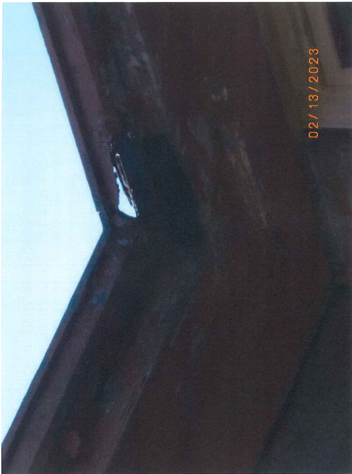
2-13-2013 3624 N 40TH ST JCR VIOLATION # 2
