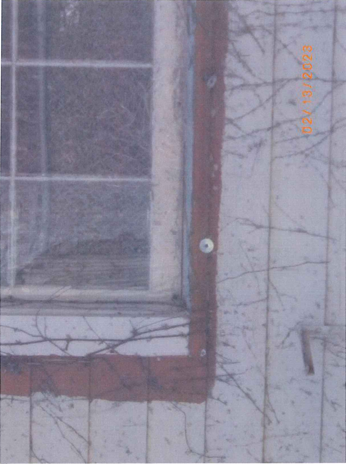
2-13-2013 3624 N 40TH ST JCR VIOLATION # 6
