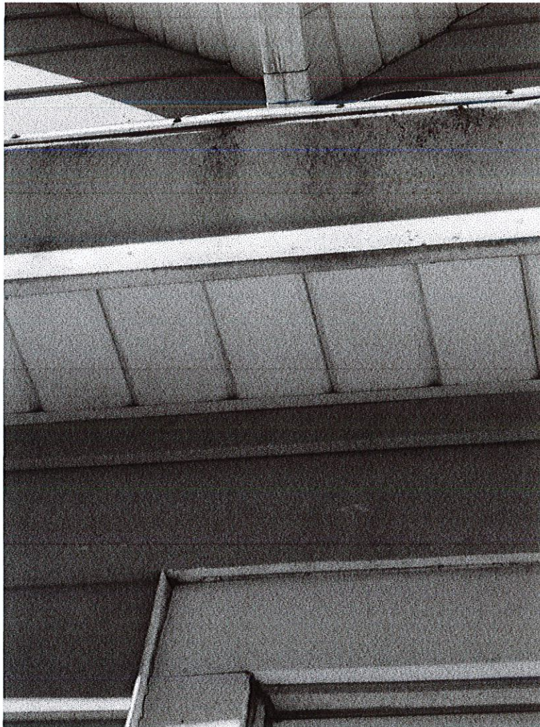
26 26-Rubber roof Date Taken: 8/13/2021 Rubber roof damaged causing the leak inside of the home.
