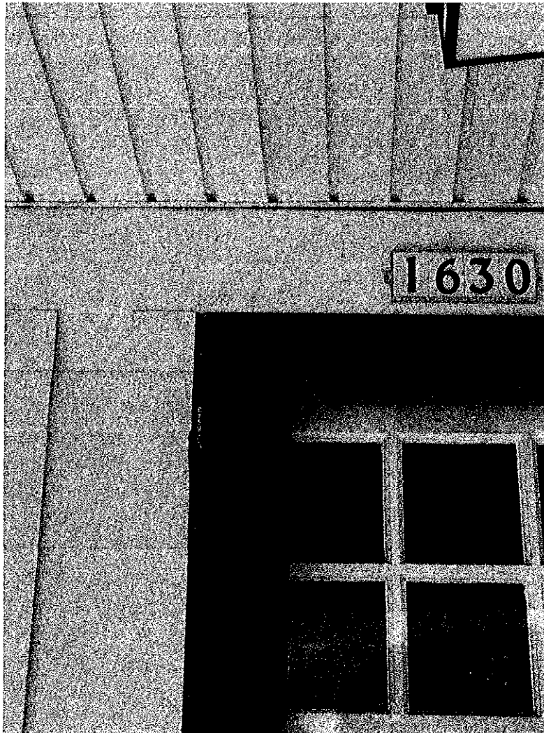
53 54-Showing the separation Date Taken: 8/13/2021 This is part of the upper deck porch.
