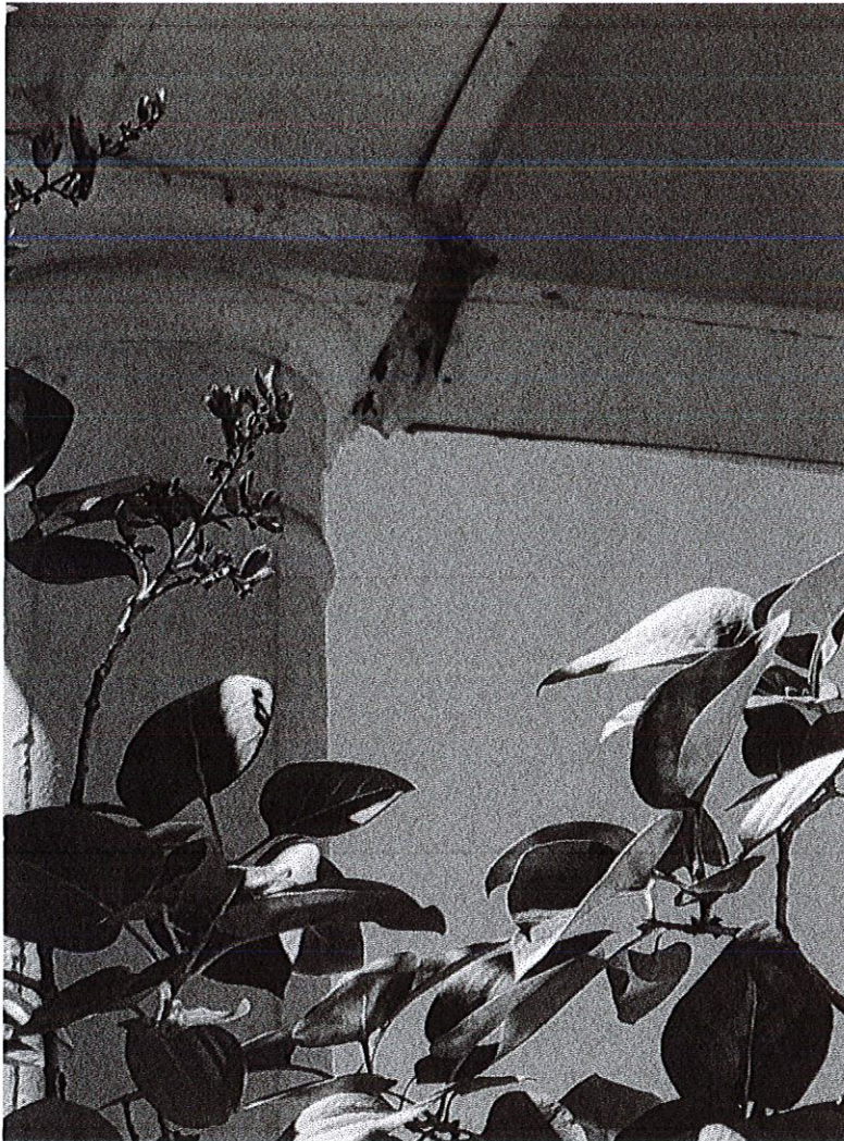
22 22-Separation of the bent gutter Date Taken: 8/13/2021
