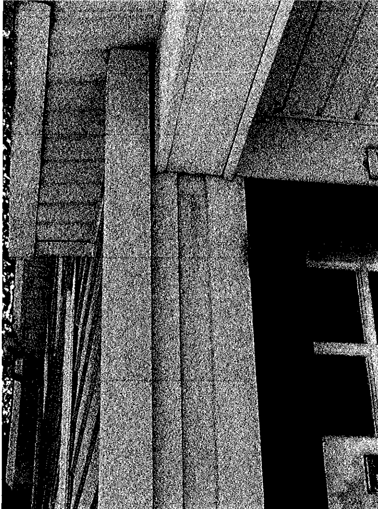
46 46-Left side Date Taken: 8/13/2021 Soffit and fascia damaged. Separation is visual here as well.
