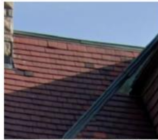
REPLACE NECESSARY ROOF TILES AND COPPER WORK FOR ROOF TO MATCH EXISTING
