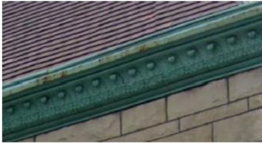
FIX / BEND / PATCH CORNICES, THEN PAINT PATCHES TO EITHER MATCH EXISTING GREEN COLOR OF COPPER OR MATCH EXISTING BROWN COLOR OF COPPER DOWNSPOUT
