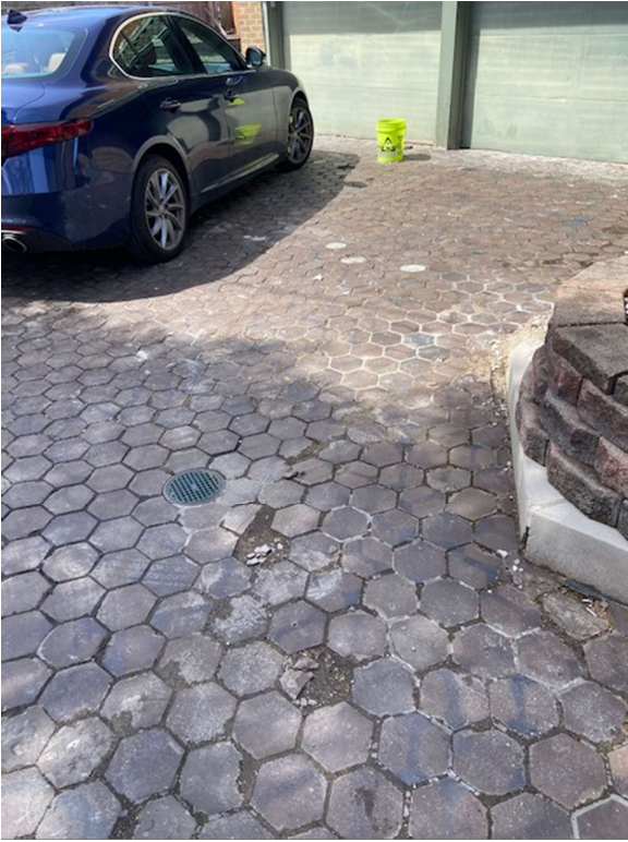
Rear Driveway – Condition Photos – showing tile deterioration:
