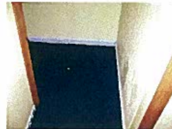
70 100_3162 6/22/2009 Taken By: Chad Frost 2222 Rec Center
