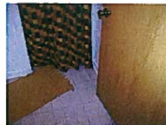
73 100_3165 6/22/2009 Taken By: Chad Frost 2222 Rec Center
