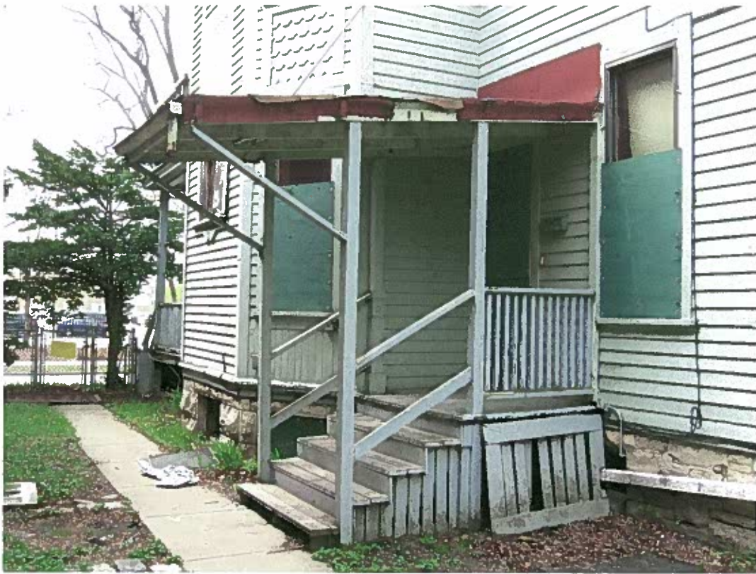
9. Side porch (North-East Elevation) with loss skirt and deteriorated roof
