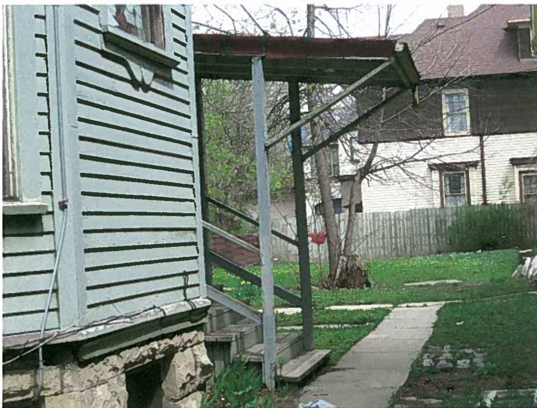
8. Side porch roof extension, undersized columns, and horizontal railings
