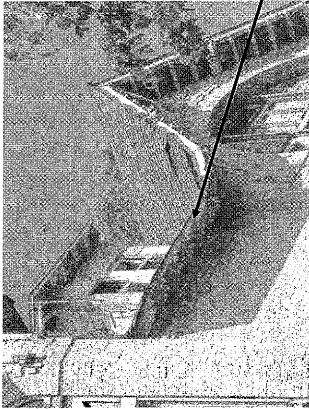
3. Closer view of roof damage on side gable taken from the south east
