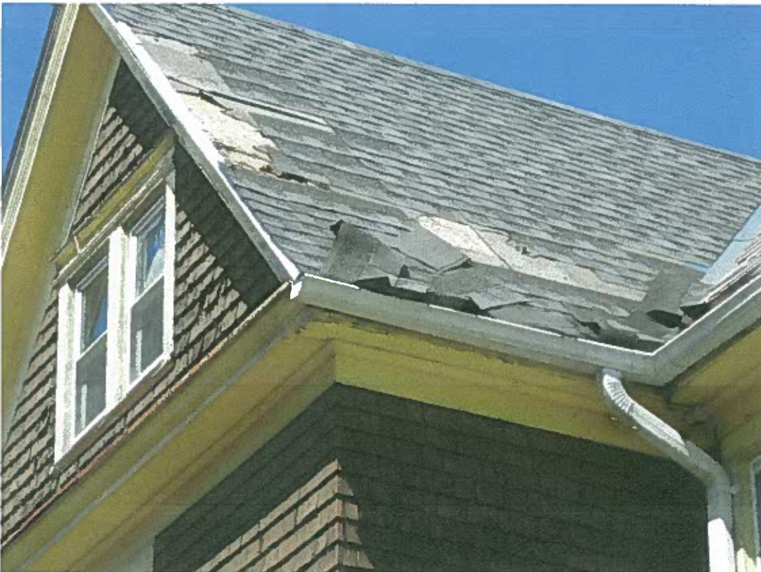
2. Side Roof on Street Front Elevation showing damaged shingles
