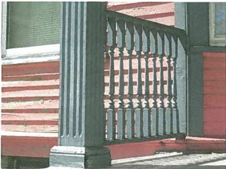
4. Front Porch south railing and column deterioration
