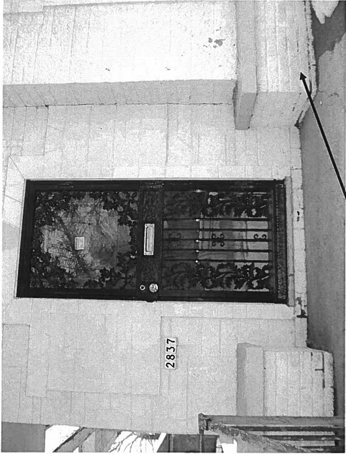
Retain front terrace walls
