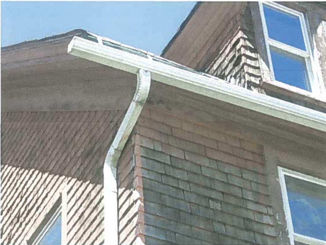
7. Second floor (South-East Elevation) cornice line connection showing new K-Style gutters and shingle deterioration
