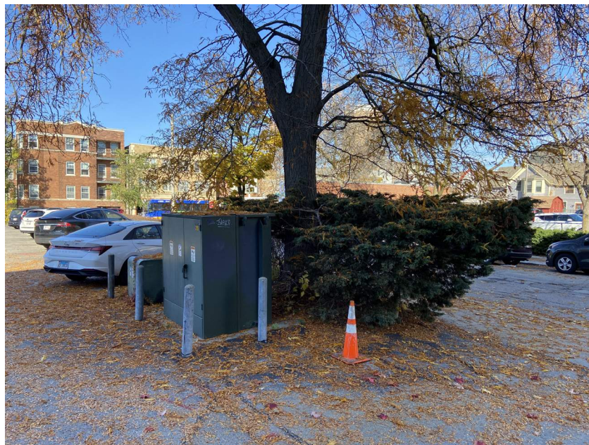
Existing electrical service to be relocated into new structure electrical vault
