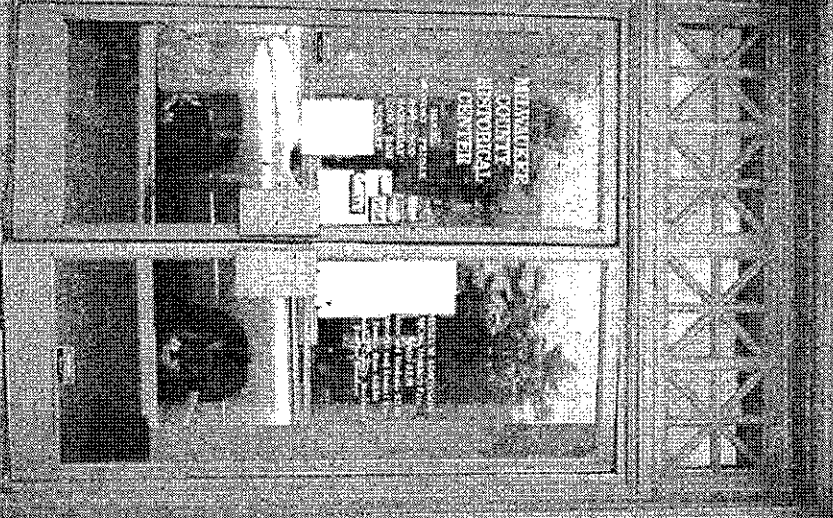
Photo no. 02 Milwaukee County Historical Center - 910 North Old World 3rd St. - Milwaukee West-side building entry - Existing condition
