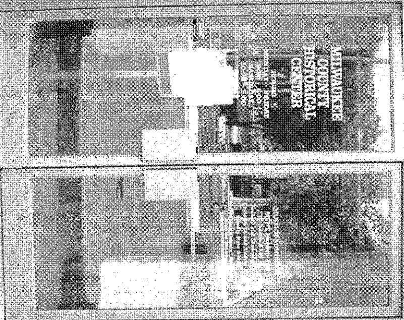
Photo no. 01 Milwaukee County Historical Center - 910 North Old World 3rd St. - Milwaukee East-side building entry - Existing condition
