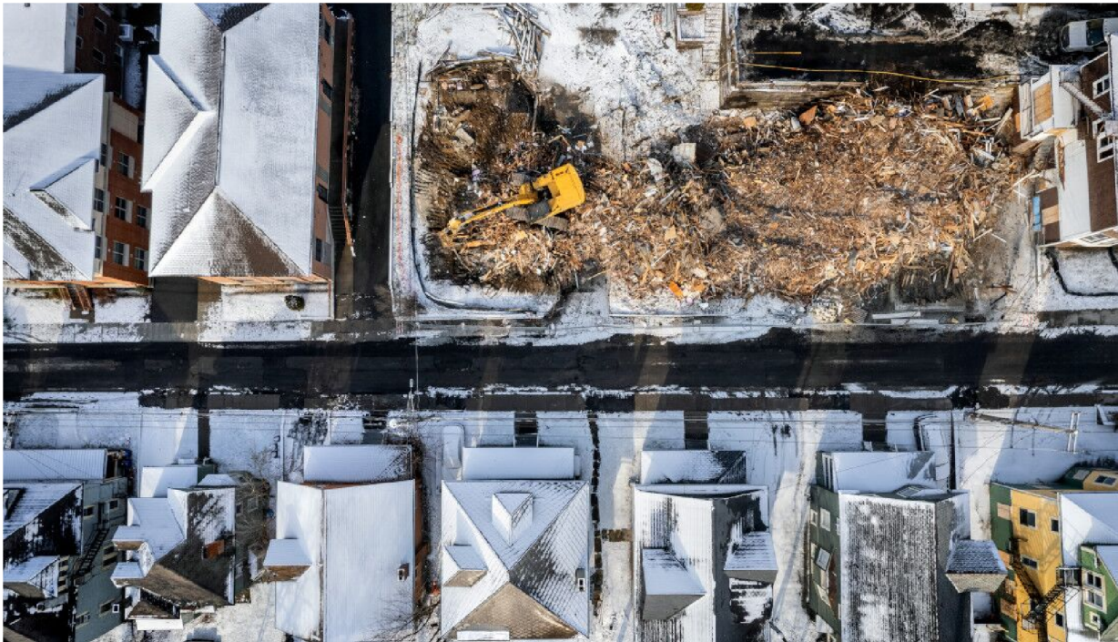
An excavator makes short work of several homes in Ithaca. Photographer: Jason Koski, Cornell University
