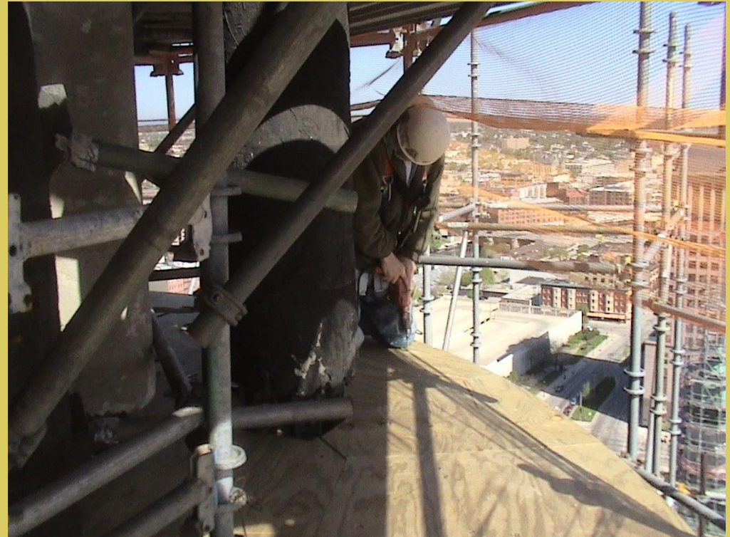
Installation of new wood decks on the lantern of the south tower.
