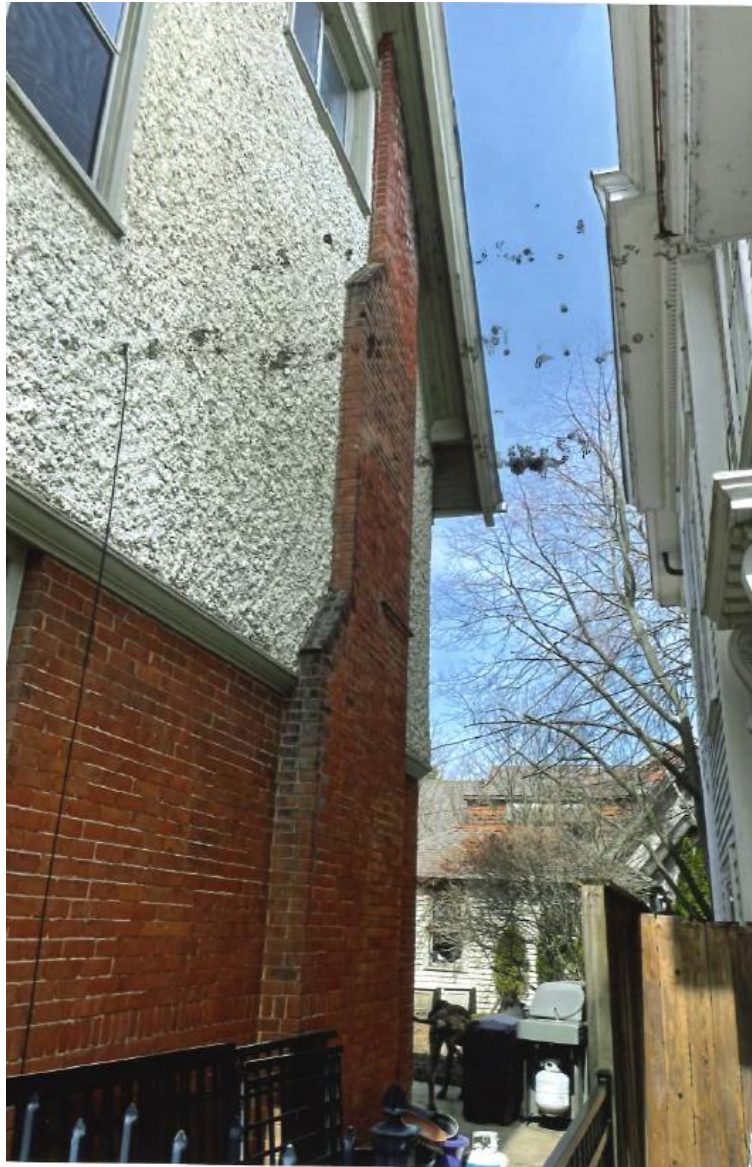
Chimney to be rebuilt
