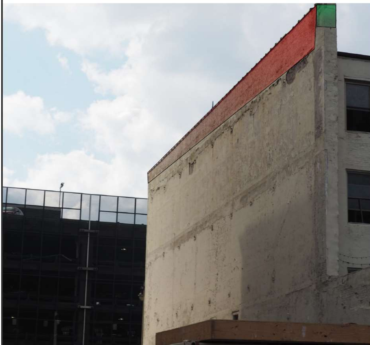
Area of repair highlighted at top of wall. Work is primarily on parapet of south wall of 514 N Water building.
