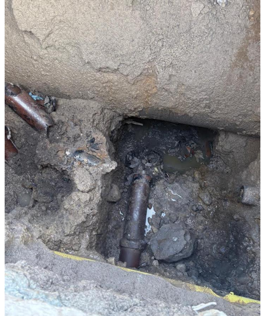
Photo demonstrating damage at 3149/3151 N. Humboldt consistent with damage in our claim - lateral compromised under the 54" main.
