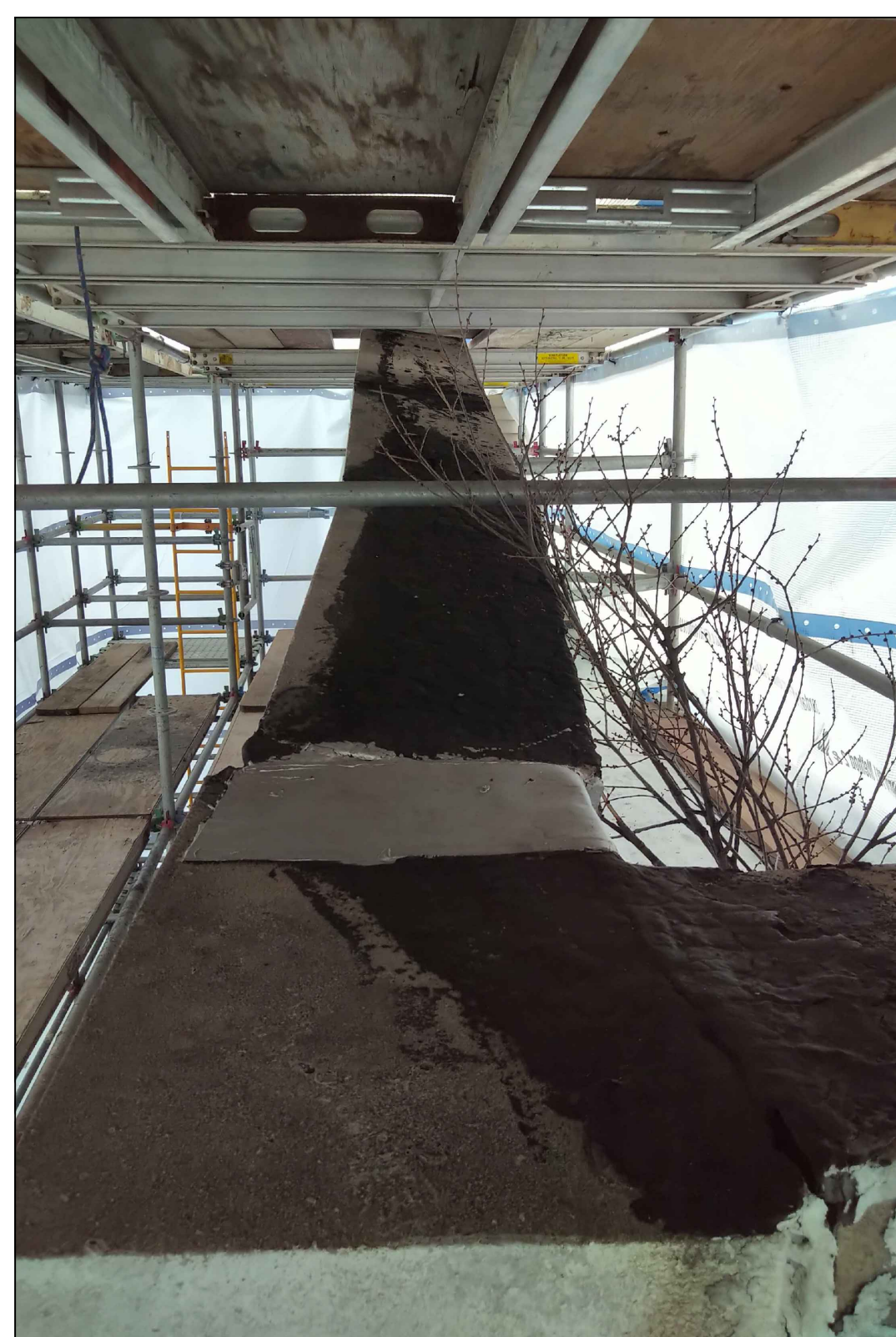
COPING STONES IMPROPERLY SEALED WITH ASPHALT
