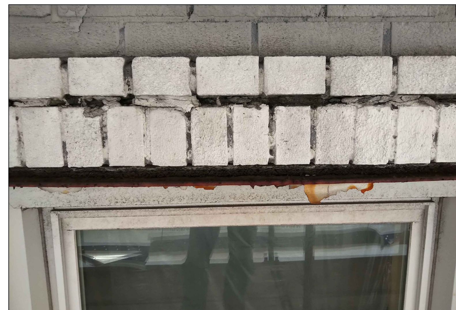
MISSING MORTAR, EXPANDED JOINTS BECAUSE OF MOVEMENT; GAP AT STEEL LINTEL NOTE THE RUST STAINS FROM THE LINTEL ON THE WINDOW
