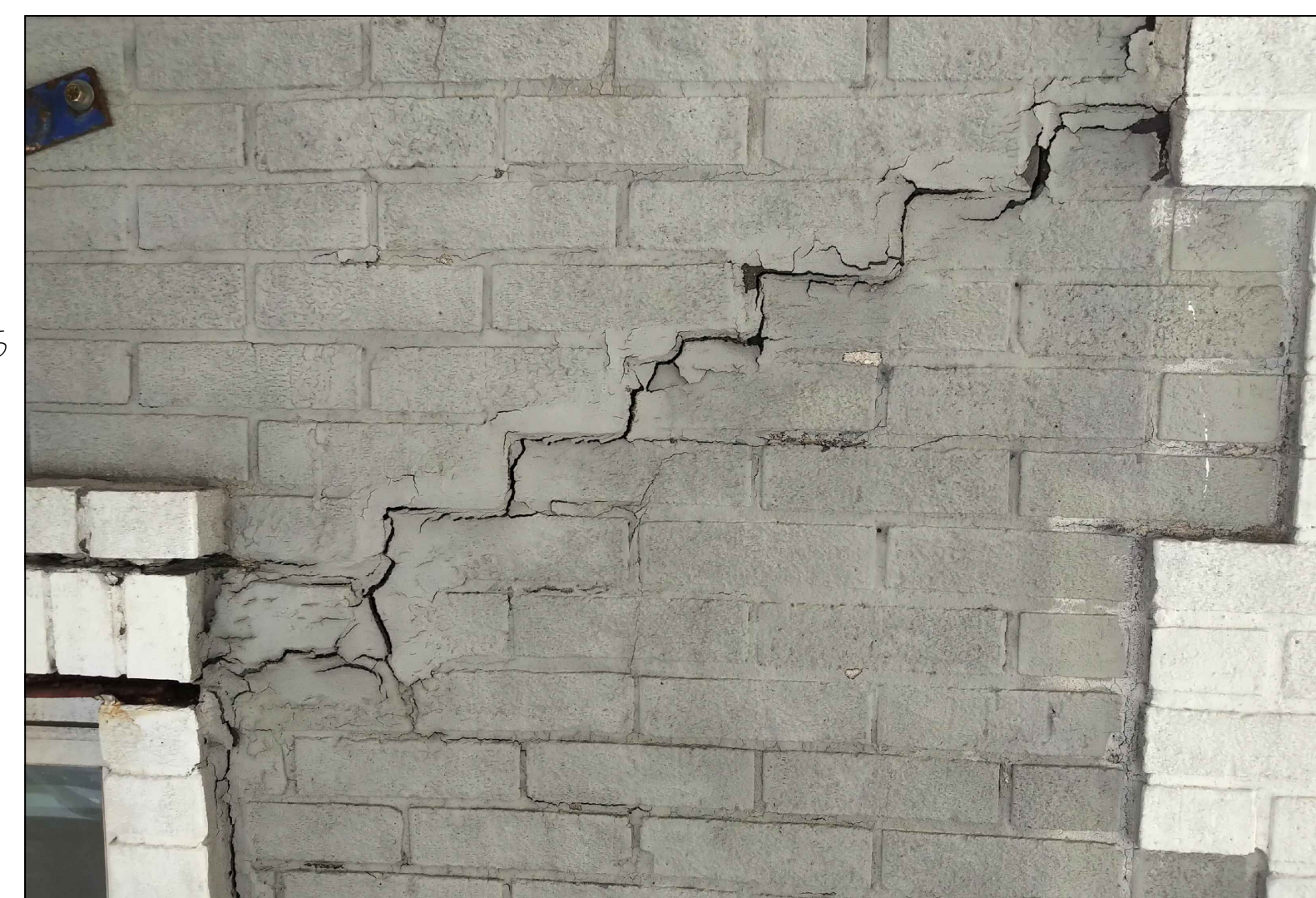
MOVEMENT CRACK FROM WINDOW LINTEL TO WEST WALL AT COIN DETAIL
