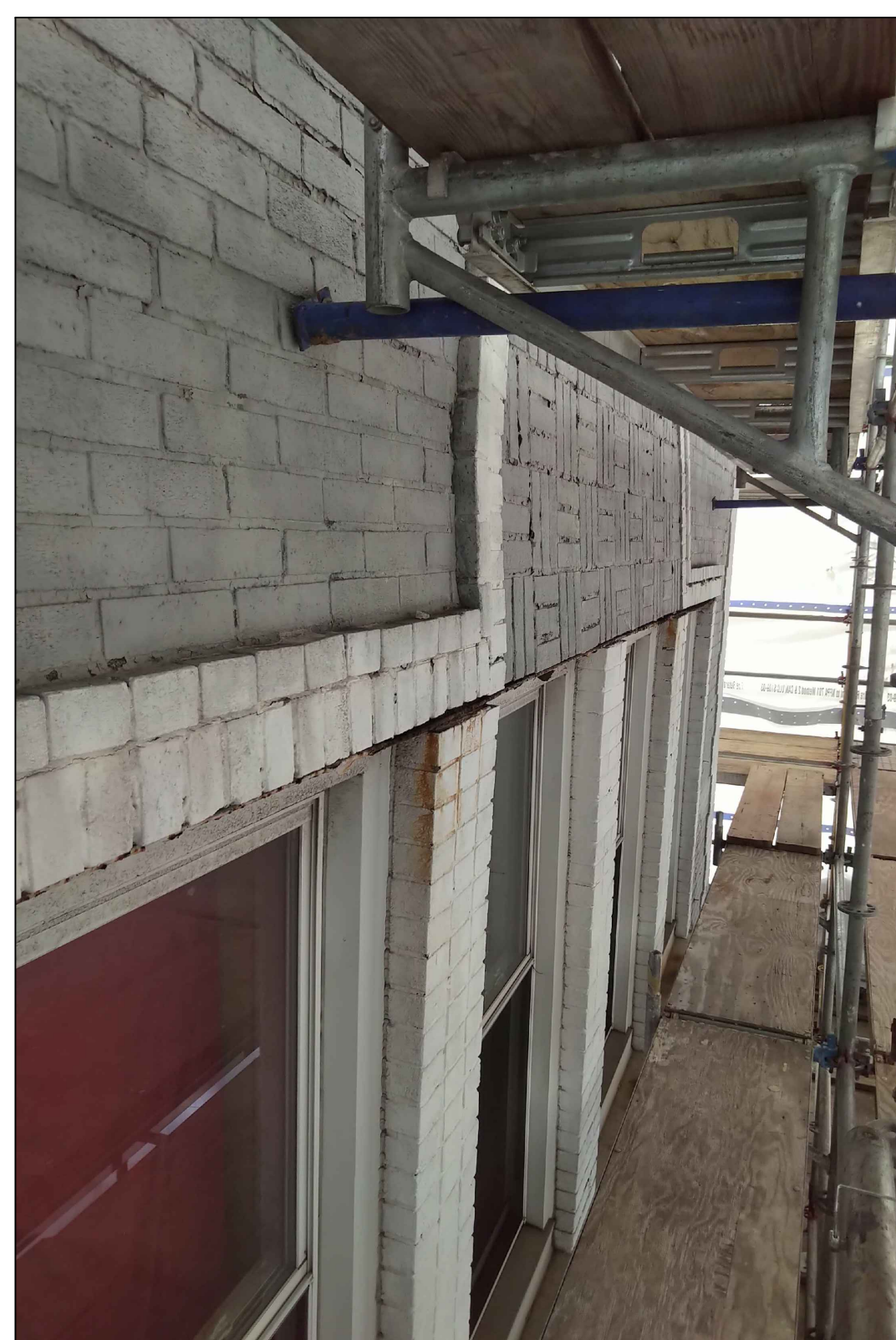
BEST PHOTO TO SHOW THE "LEANING" OF THE UPPER PORTION OF WALL. AT LEAST 5 DEGREES OUT OF PLUMB
