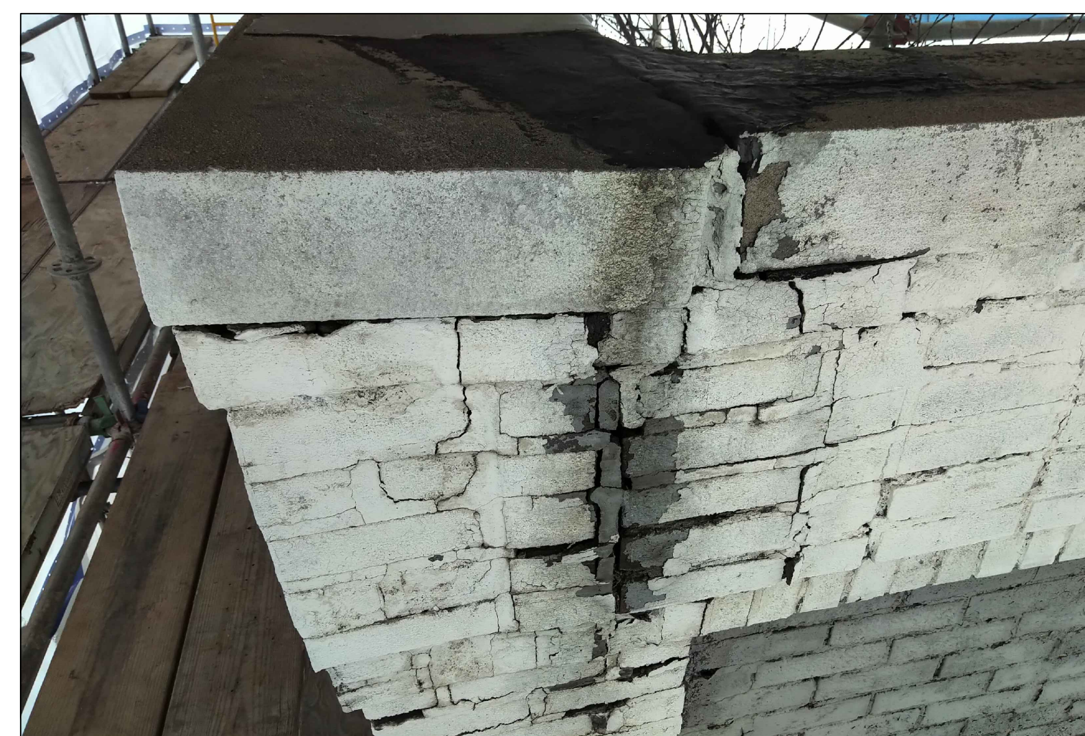
UPPER WEST CORNER DETAIL - WATER INFILTRATION DAMAGE BRICK AND COPING MOVEMENT - POOR JOINT REPAIR
