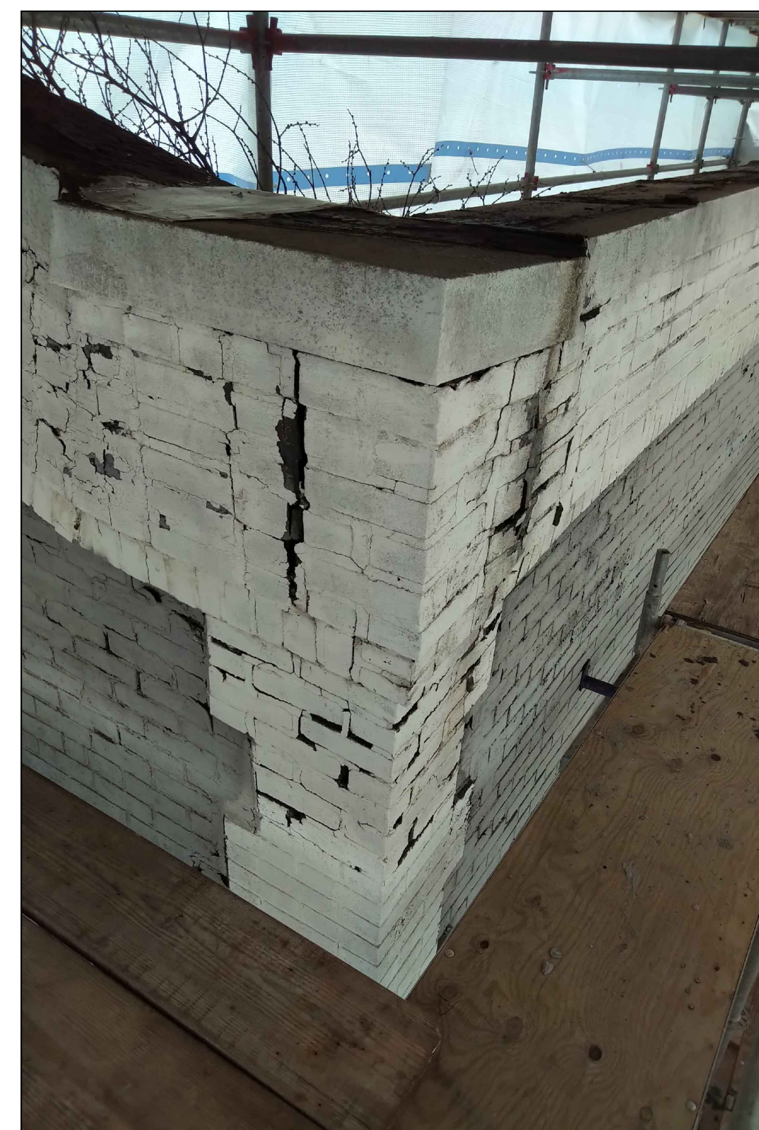
UPPER WEST CORNER DETAIL - WATER INFILTRATION DAMAGE BRICK AND COPING MOVEMENT
