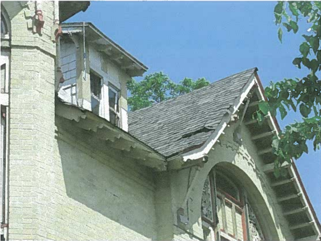
3. Closer view of roof damage on side gable taken from the south east
