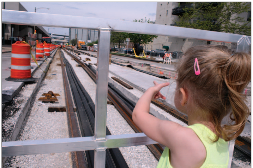
▲ Further west on St. Paul Avenue construction progressed enough that it was starting to resemble a streetcar Line. Gracie, then 2-½ years old, was visiting Grandpa who took her along on May 22, 2017. Standing on one of the pedestrian bridges to walk over the construction, Gracie pointed to the westbound track and said "train." In September 2018 Gracie and Grandpa attended the press conference at the car barn when Milwaukee Mayor Tom Barrett was announcing opening day. Every time the mayor said "Hop," Gracie would hop. Noticing this, Mayor Barrett called Gracie up to the podium to hop every time he said "Hop." She appeared in all the television newscasts that evening.
