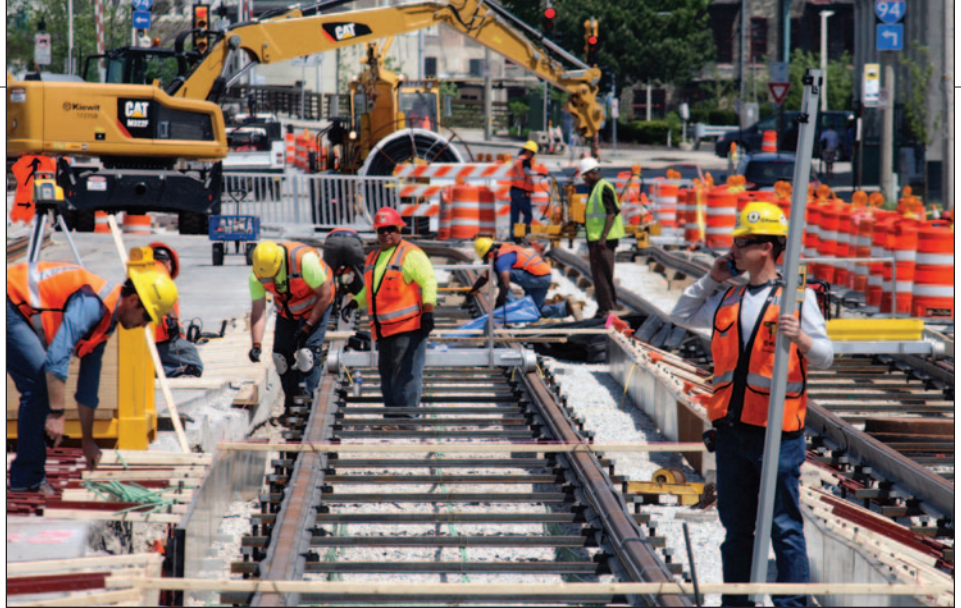
▲ On May 18, 2017, construction was underway on St. Paul Street. We are looking east from Second Street toward Plankinton Avenue.
