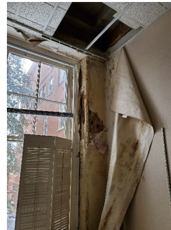
Photo 20: Deteriorated walls and window.
