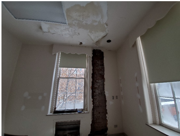
Photo 19: Deteriorated wall and ceiling in Northwest Quadrant.
