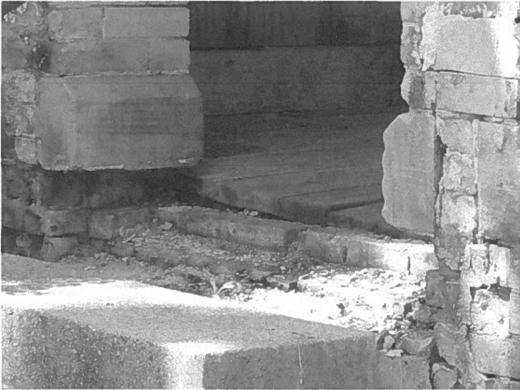
15. Close up view of missing threshold on northeast side porch
