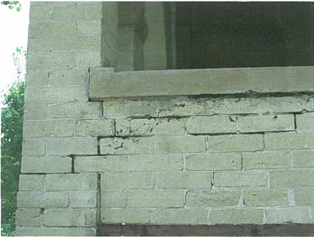
17. North wall of northeast side porch showing a need for tuckpointing
