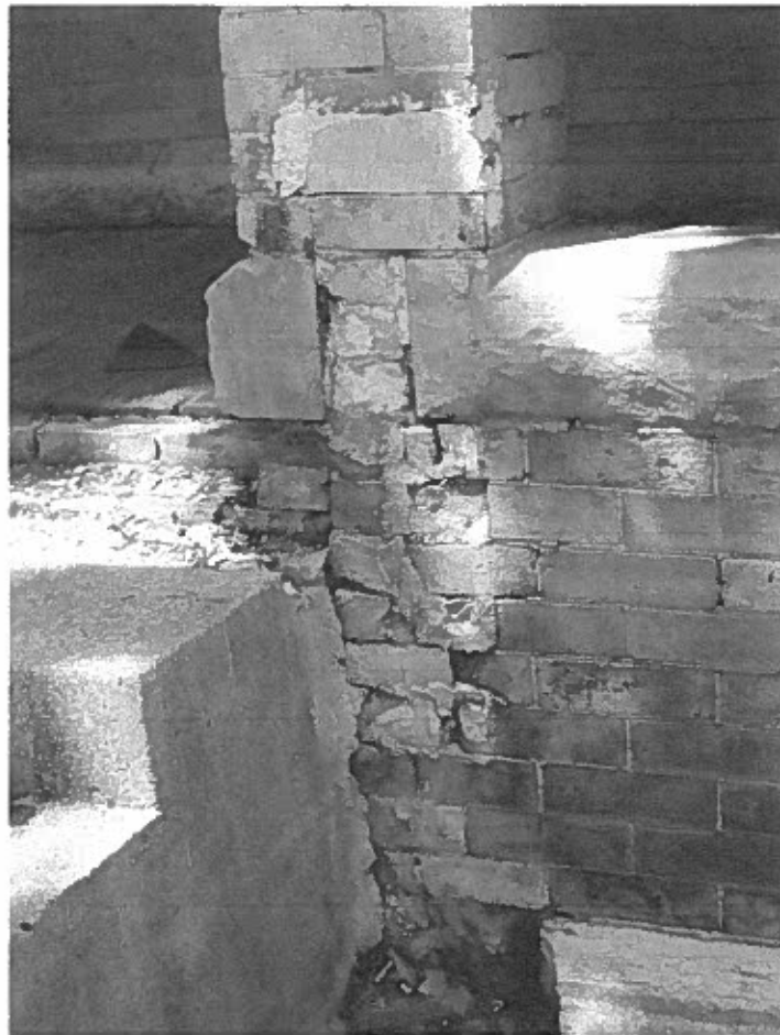
16. Wall deterioration on north side of northeast side porch
