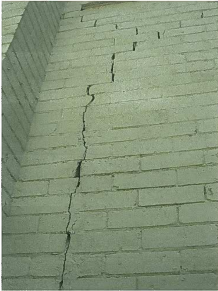
19. Existing crack in the west wall of the house
