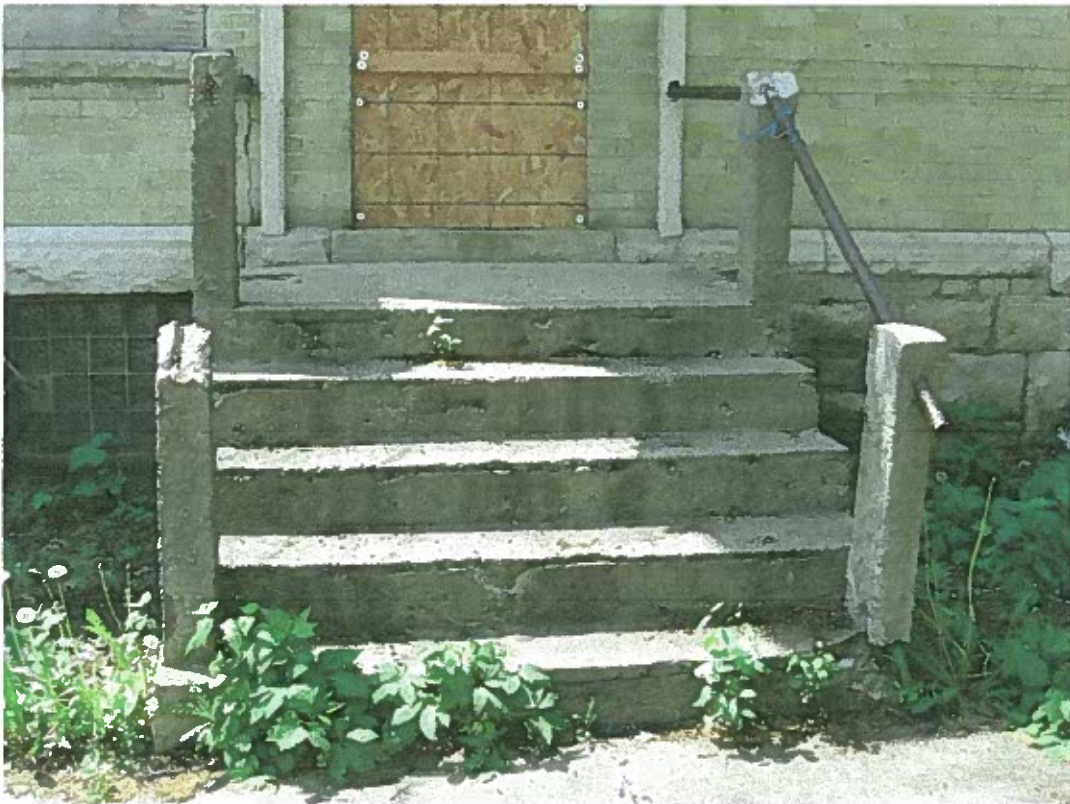
18. North elevation rear entrance porch deck with stair and railing deterioration
