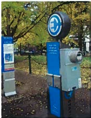
Electric car charging station on a public street in Portland, OR
