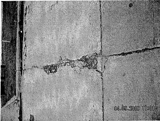
Photo of spalling at a rigid (Portland Cement-Concrete) joint
