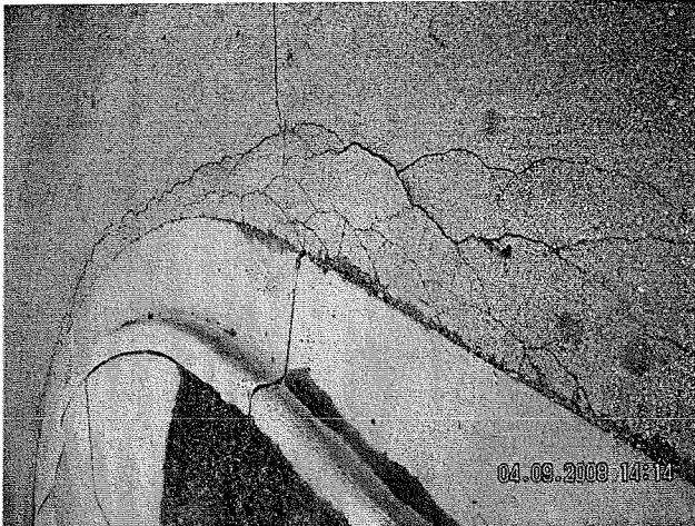
Photo of Alligator Cracking at the edge of pavement
