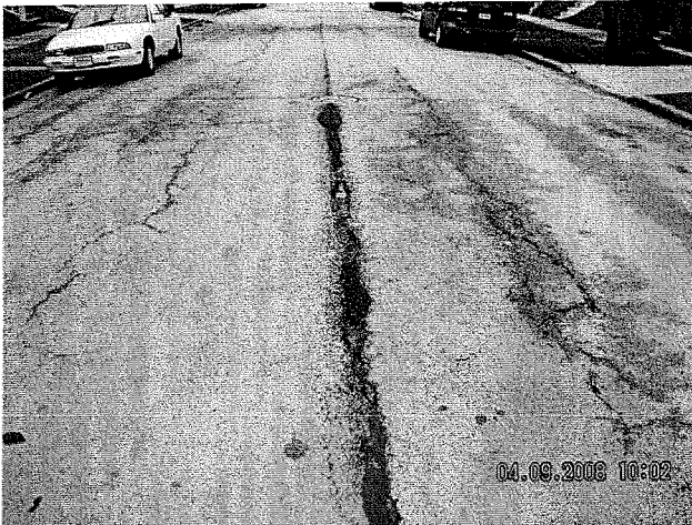
Photo of deteriorated construction joint
