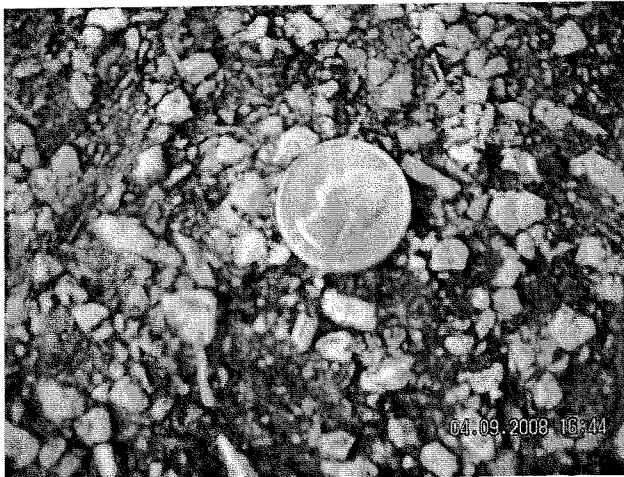
Photo of Stripping / raveling
