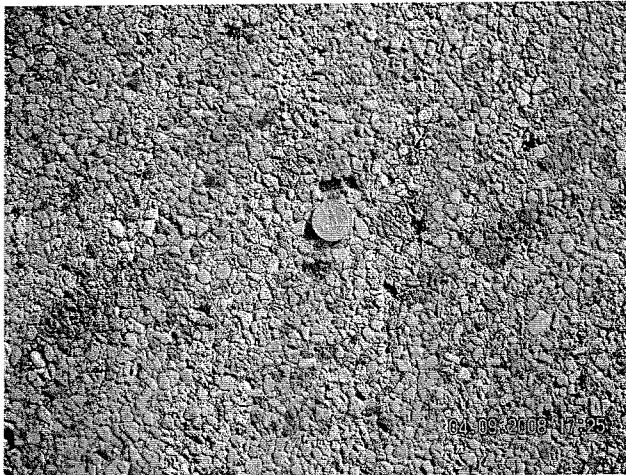
Photo of Pitting
