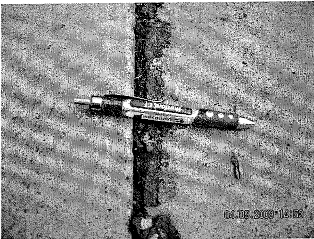
Photo of faulting
