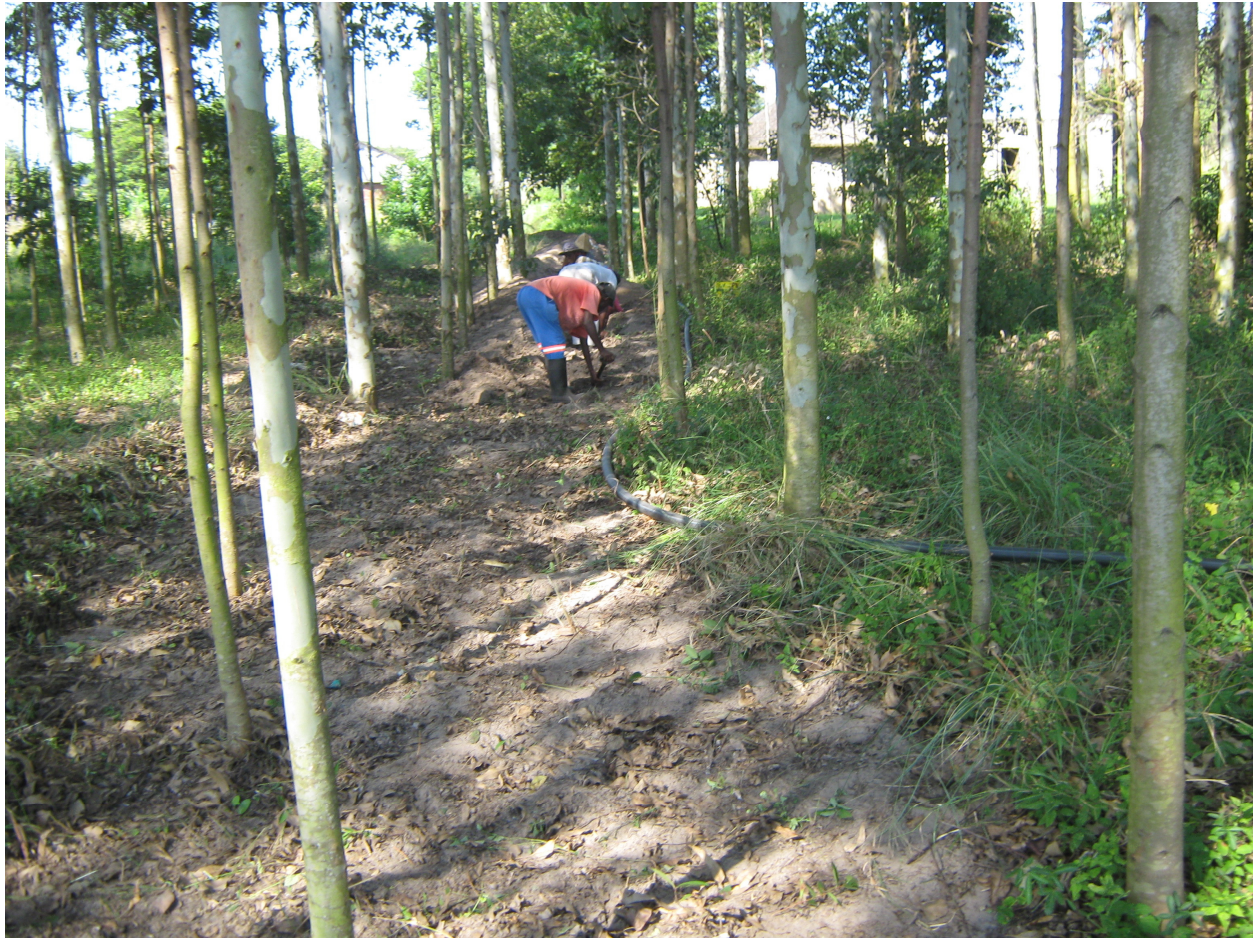
Women clearing the pipeline route where the water pipeline will be installed
