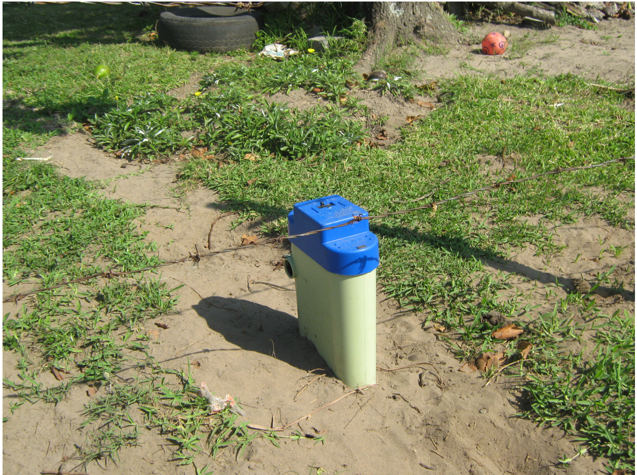
Water meter is installed ne xt to the boundary fence of the household
