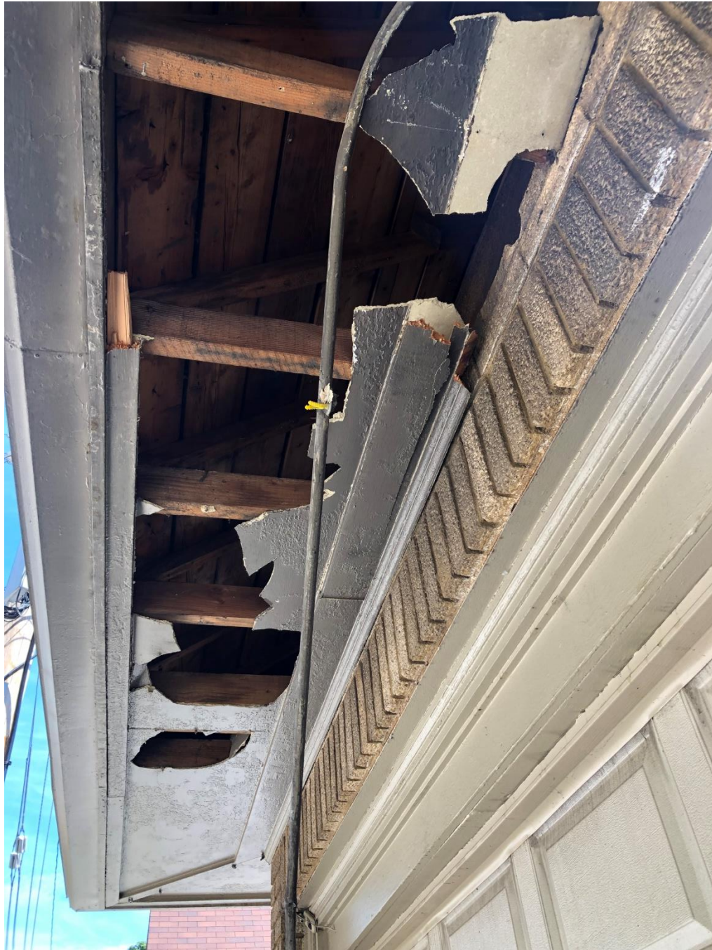
Representative damaged area.
