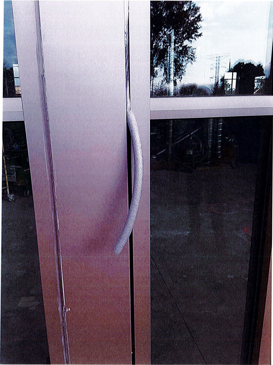
Backer rod and caulk need to be completed, several locations.
