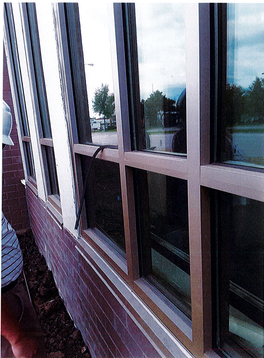
Gaskets loose / not installed properly in several locations
