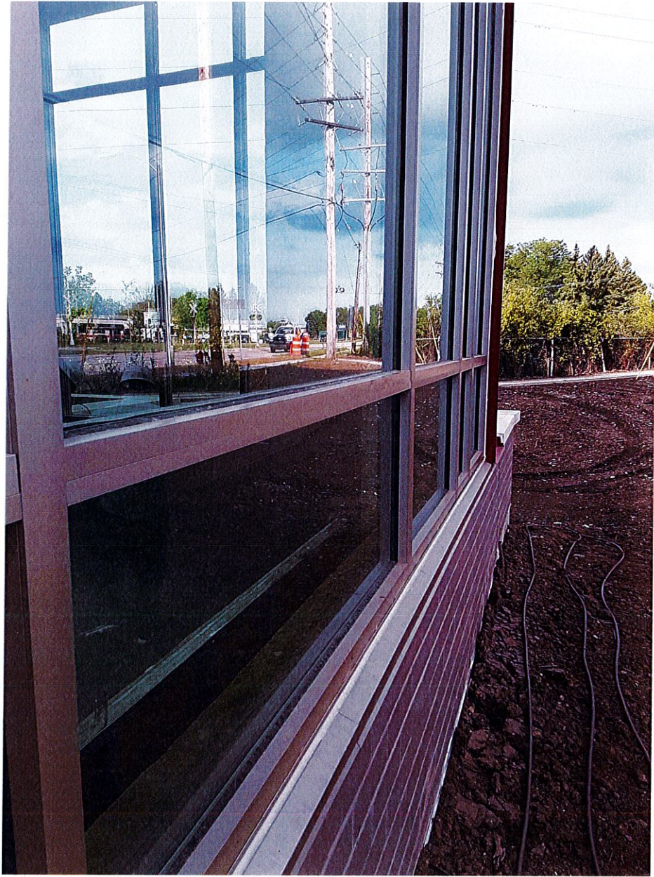
Dented mullion on north façade near NW corner needs to be replaced
