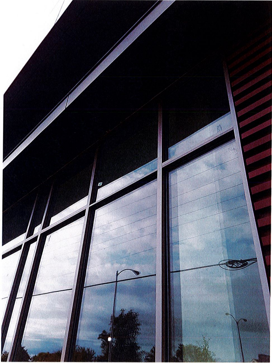
Soffits not installed multiple exterior locations
