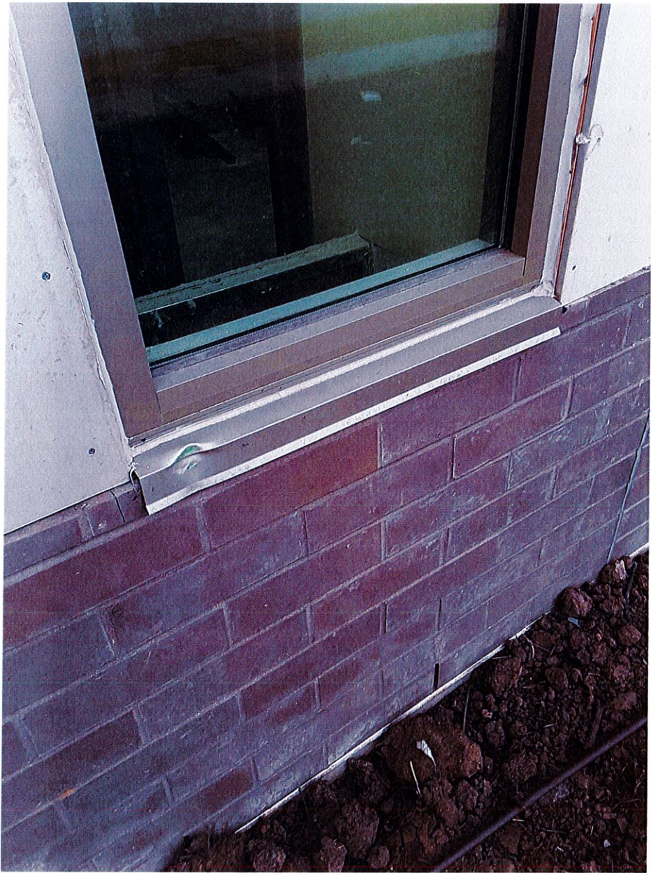
Base flashing dented and needs to be replaced, several locations
