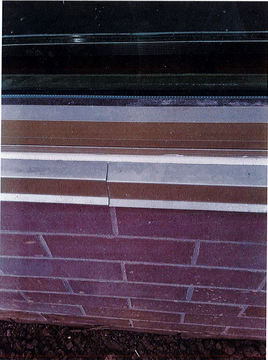
Base flashing jointing not aligned properly, several locations
