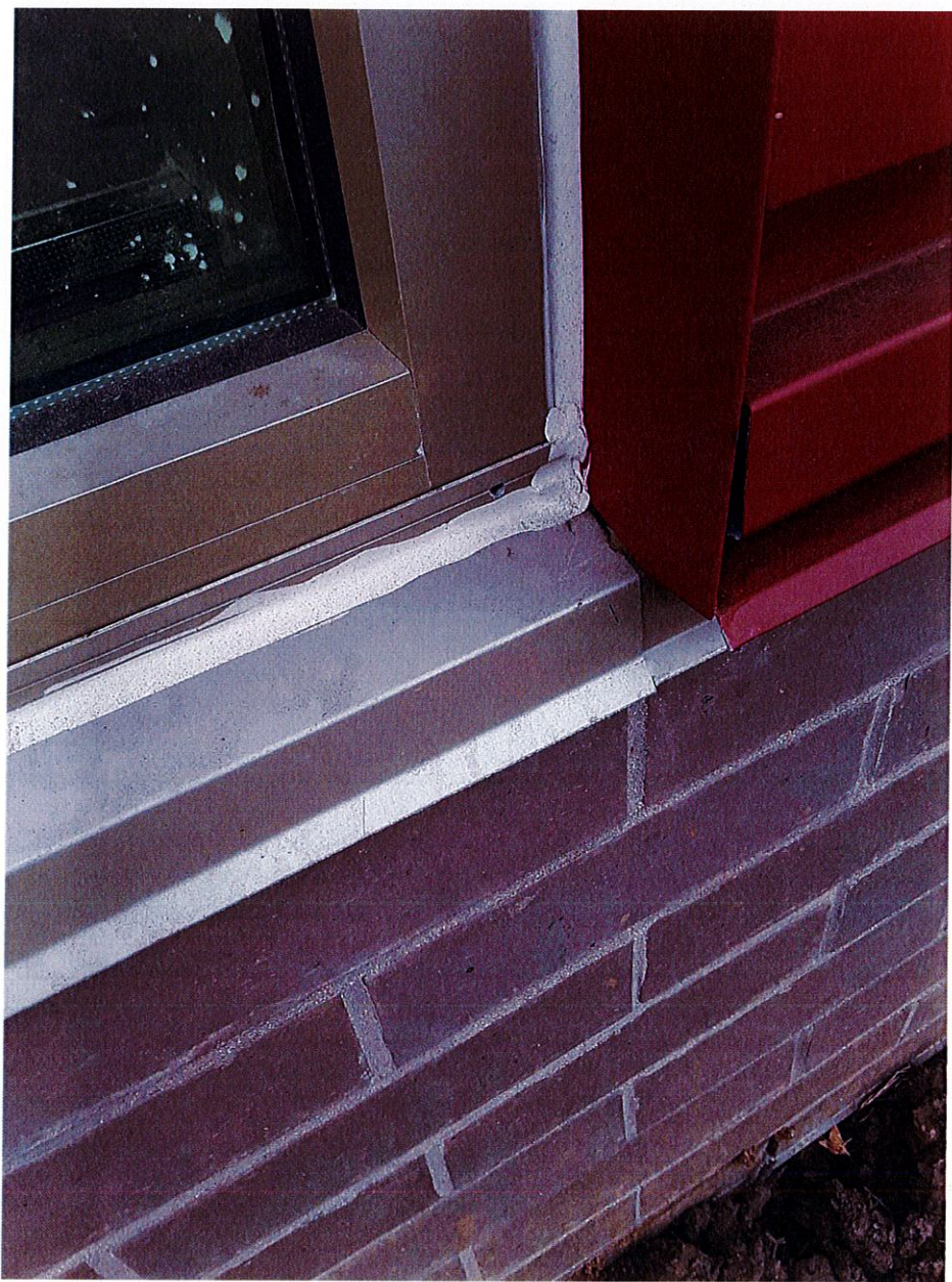
Workmanship of caulking is unsatisfactory, several locations
