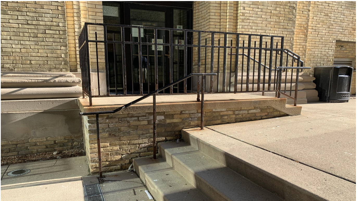
Exhibit F Existing railing and stair located in Cathedral Complex. New railing, ramp, and stair details to be similar.
