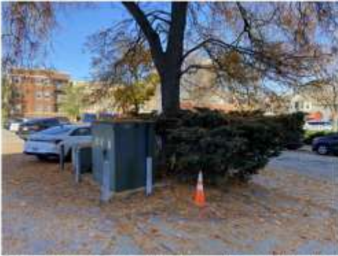
Existing electrical service to be relocated into new structure electrical vault
