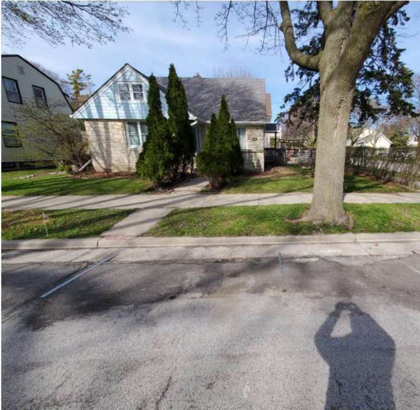
set 3: test drill holes 10/1/21 in front of house where leak found 12/3/21
