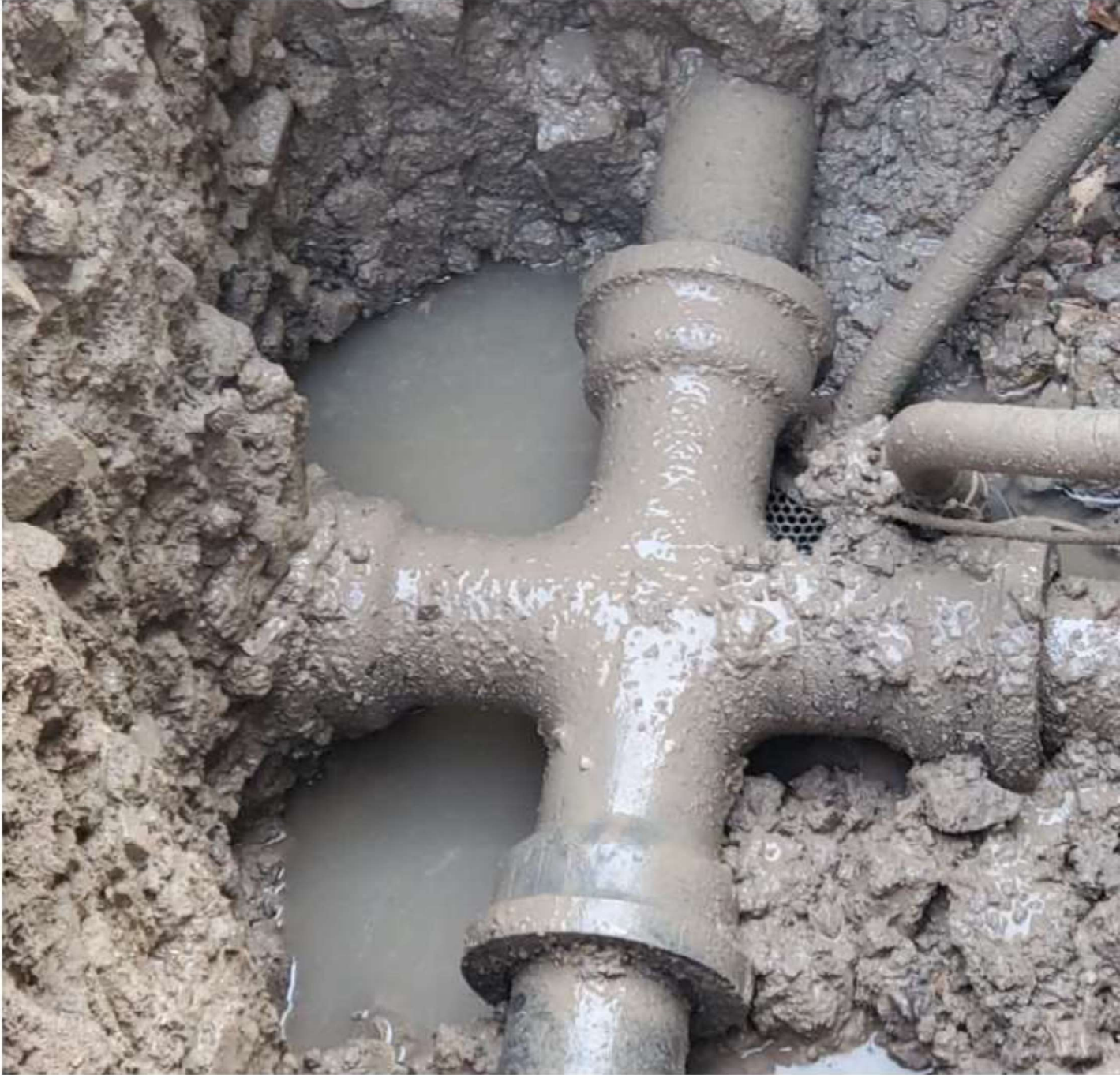
set 3: 10/1/21 4 water mains at my corner
