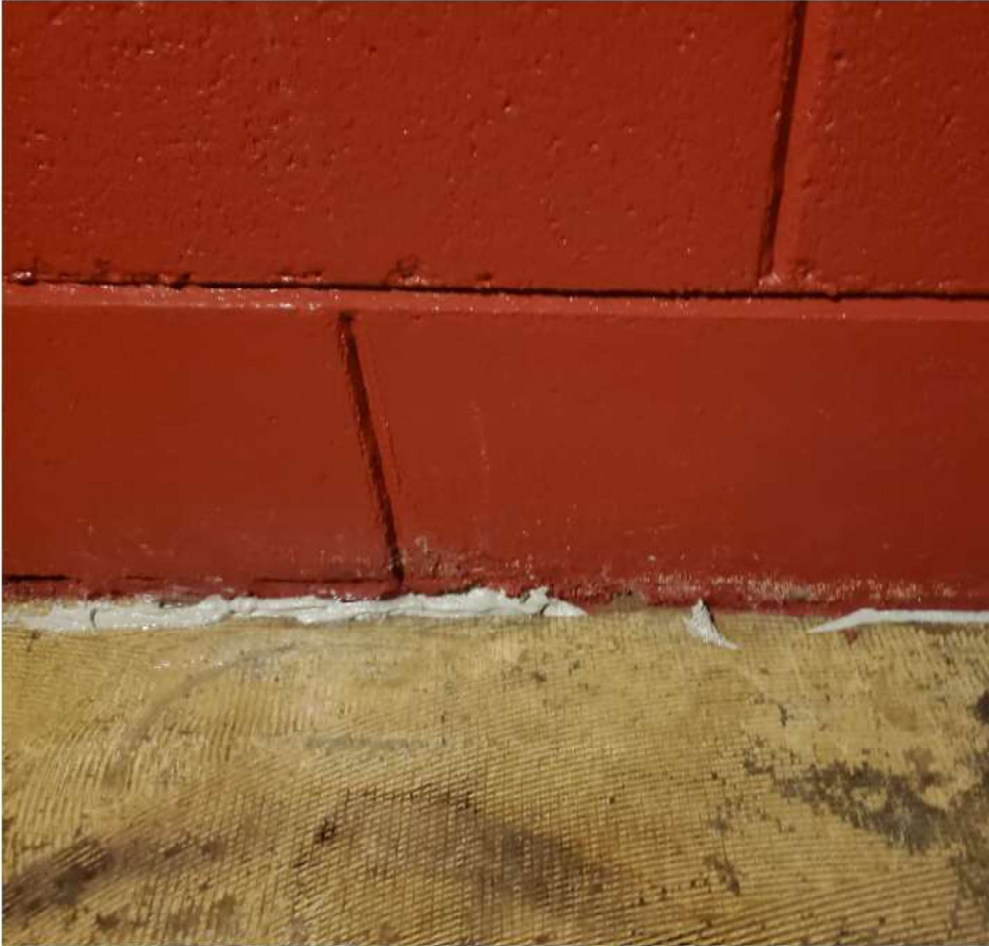
set 1, 9/18/21, failed caulking
