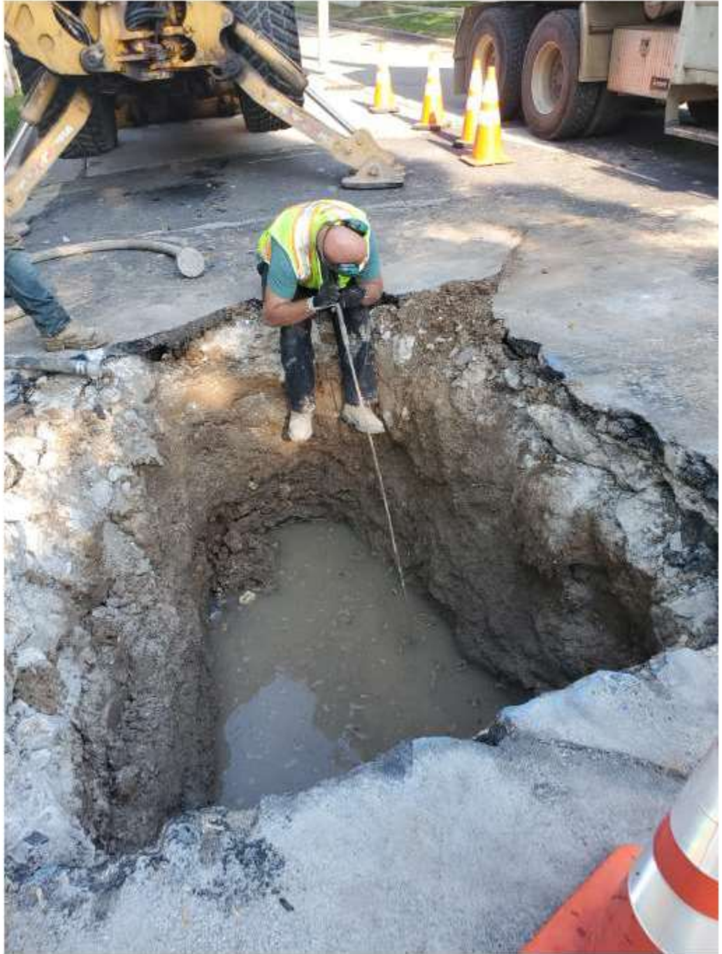
set 3: Oct 1 my corner, listening for hiss of leak through water filling up quickly
