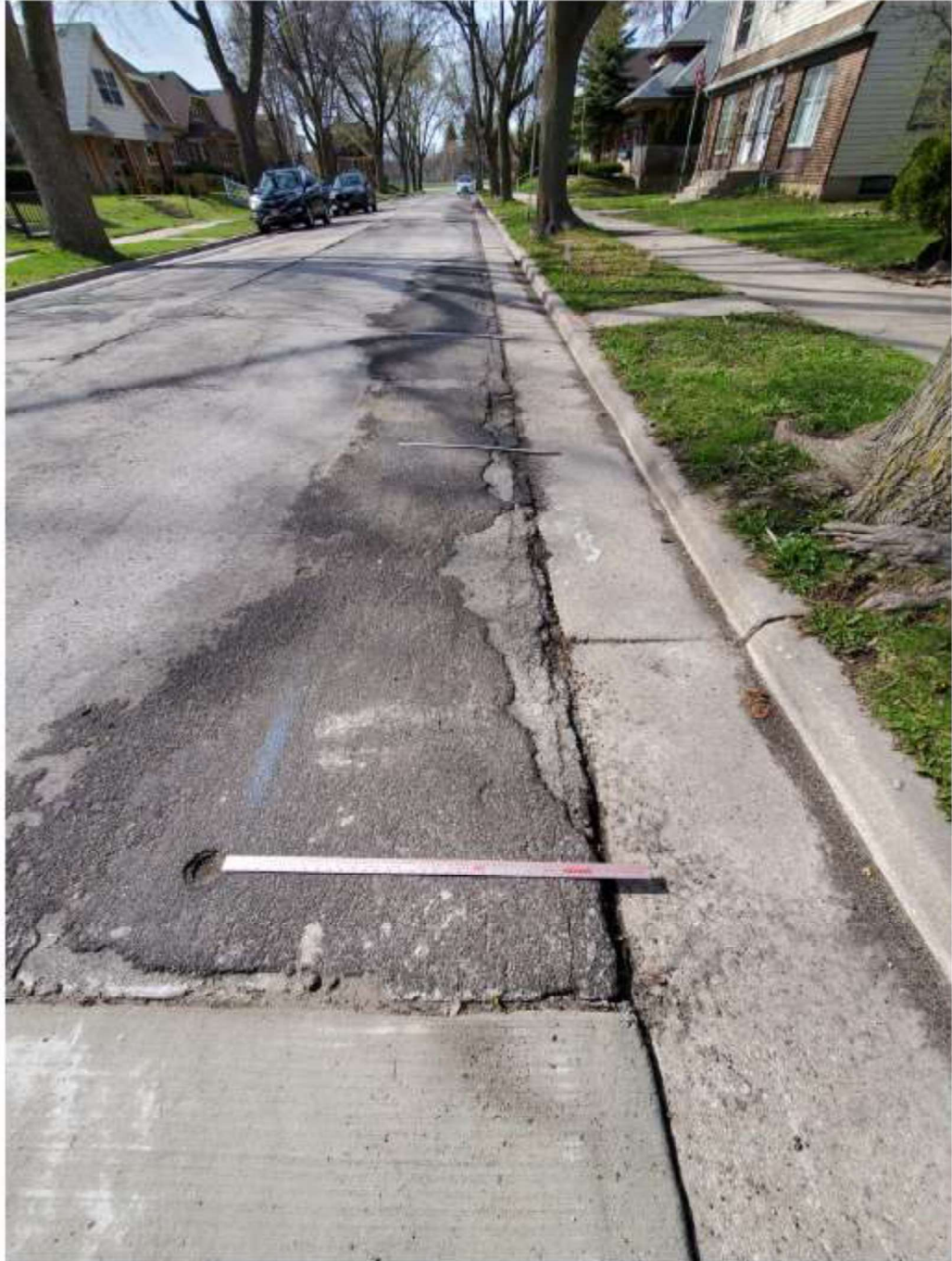
set 3 new cement at bottom where main leak fixed 12/3/21 asphalt is from previous patch
