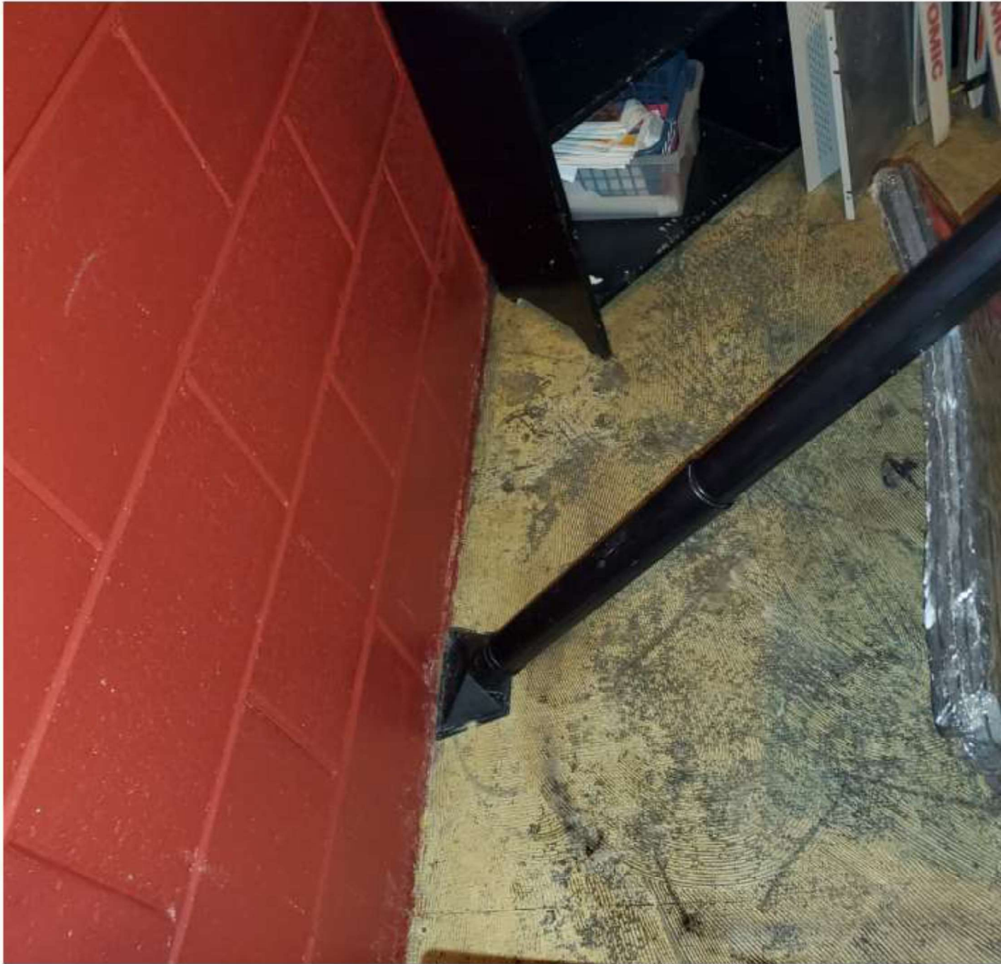
set 1 9/18 vac at trickle leak
