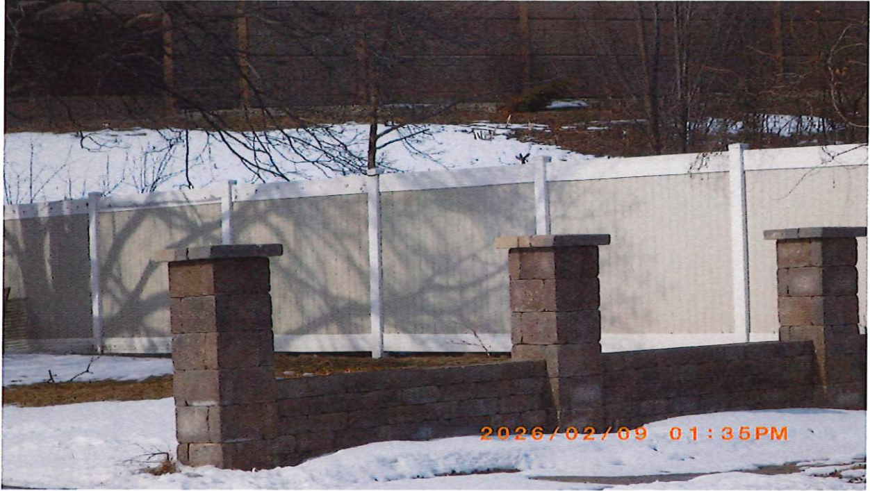
3263 S 3rd Street. (2/9/2026) (G. Armstrong/ Special Enforcement) (ORD-25-03604. Violation #3)
