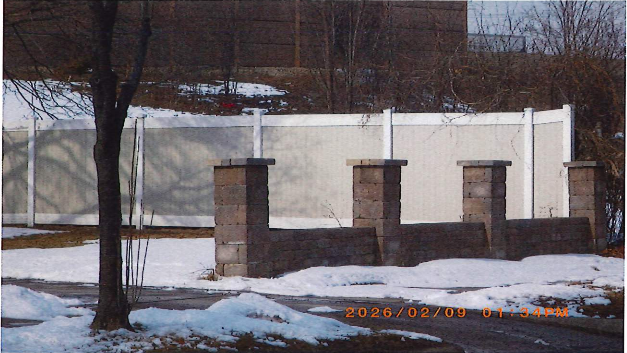
3263 S 3rd Street. (2/9/2026) (G. Armstrong/ Special Enforcement) (ORD-25-03604. Violation #2)
