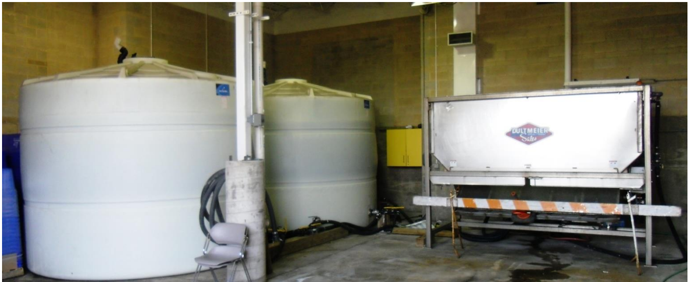
City of Milwaukee DPW salt brine maker and holding tanks
