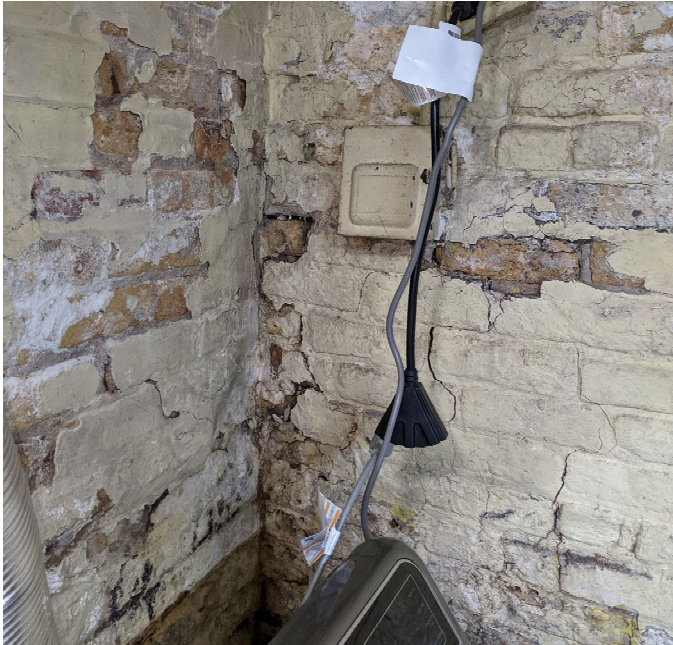
View of NW foundation corner. Both walls are bowed over 2" from excessive lateral pressures.
