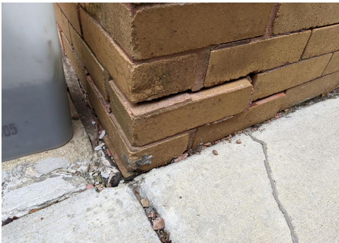
Exterior NW corner brick damage and movement along displaced foundation walls.
