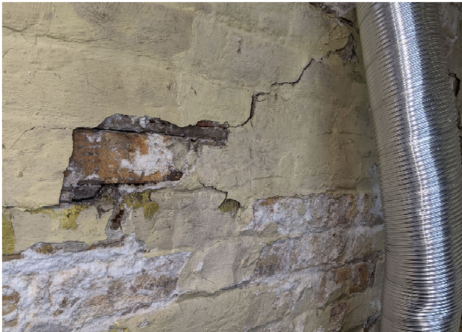
View of wall cracks and deterioration along west foundation wall.
