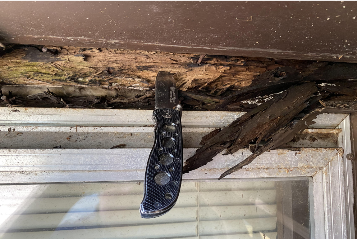
Photo 9 - Damaged Wood Header Above First Floor Windows
