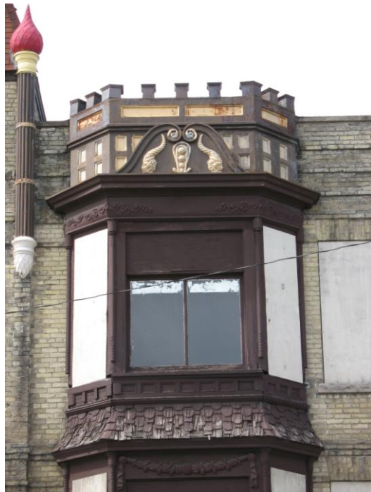
HUMMEL / UIHLEIN BUILDING 2673-2679 N. MARTIN LUTHER KING JR. DRIVE HISTORIC DESIGNATION STUDY REPORT APRIL 2010
