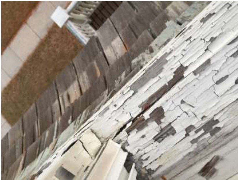
Detail of typical damage
