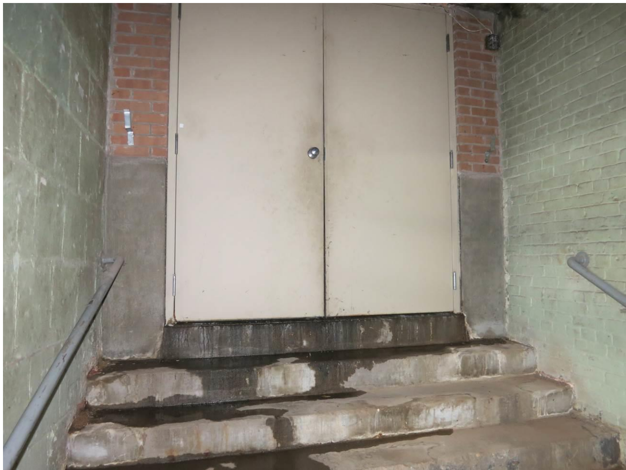
Exterior doors to Stair 8 from the inside. The poured concrete stair and surrounding construction seen here will be demolished in the foundation reconstruction. Stair does not meet current code. The pair of entrance doors swing into the space and a landing is required on both sides of the door.
