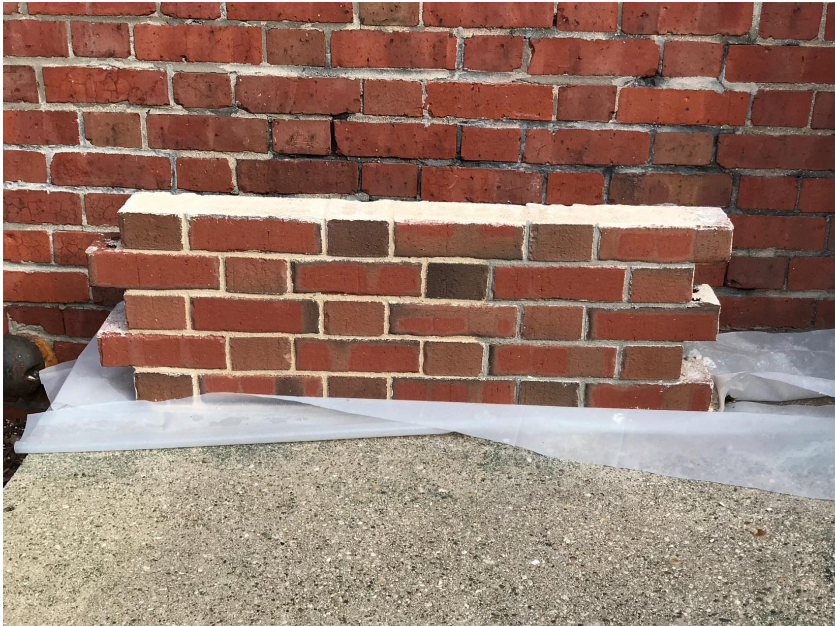
Two color mortar test panel. Sandy color at left is to be used. Also showing typical wall condition with mismatched mortars from previous attempts at repairs.
