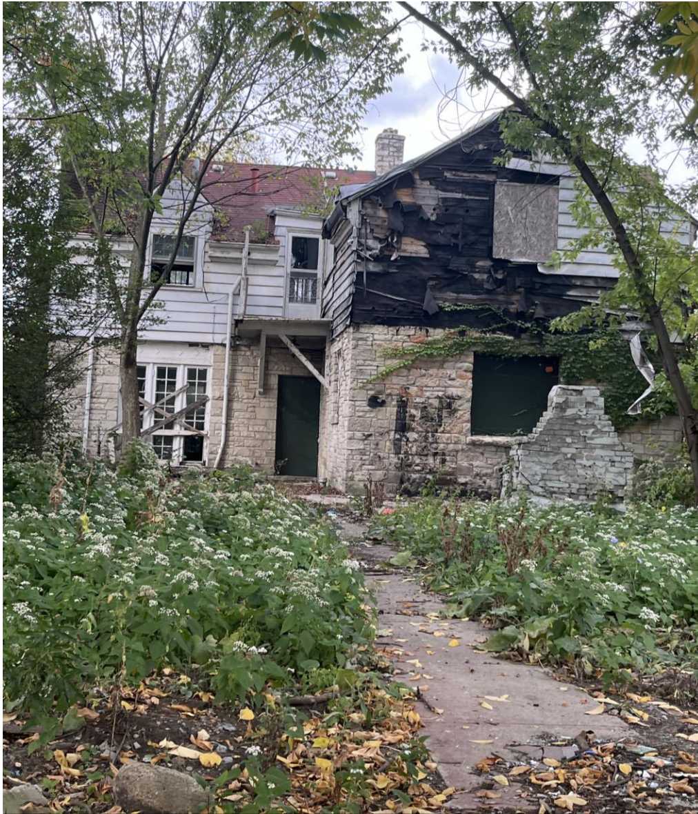
Existing conditions post-fire
