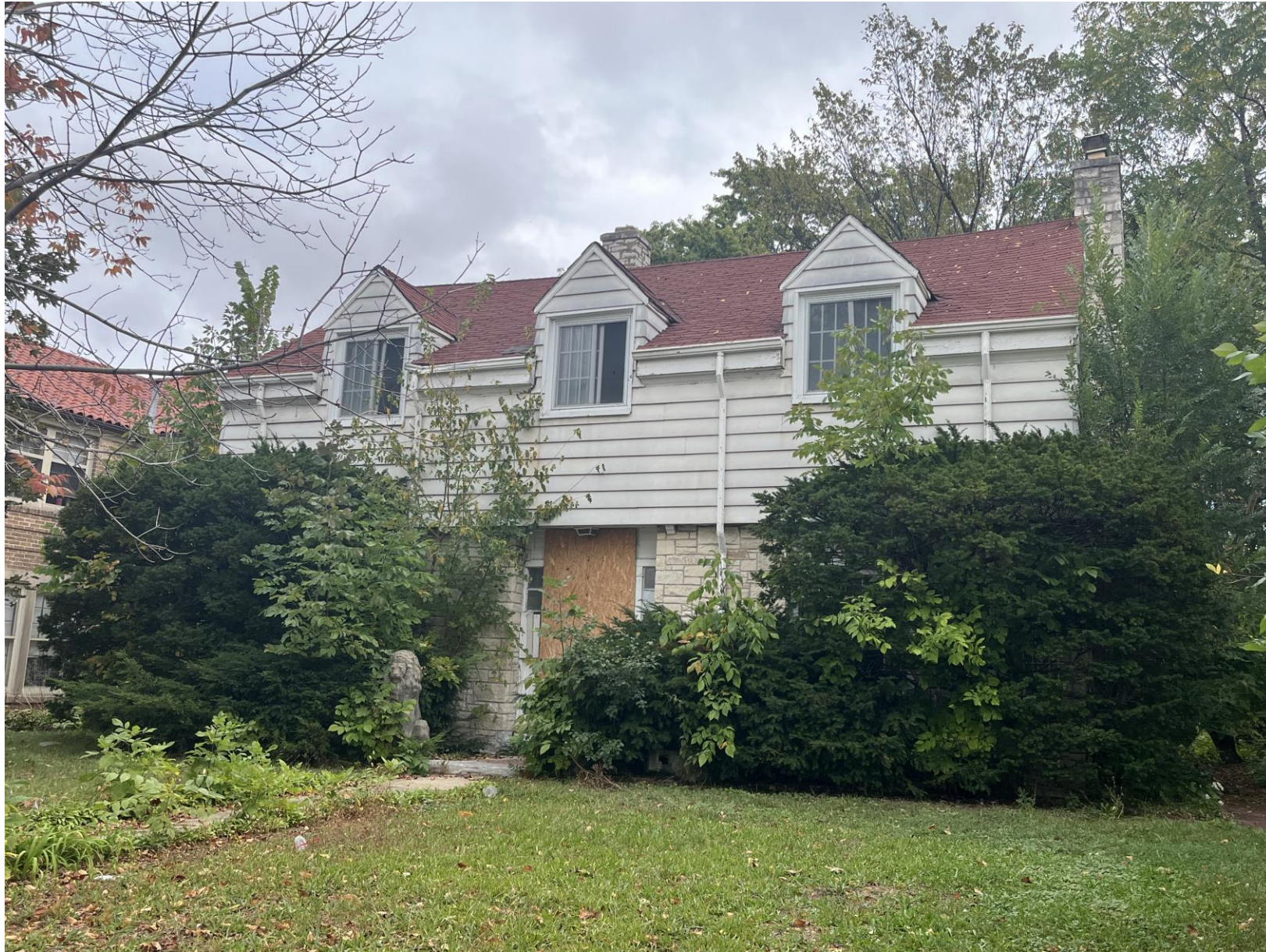
Existing conditions post-fire
