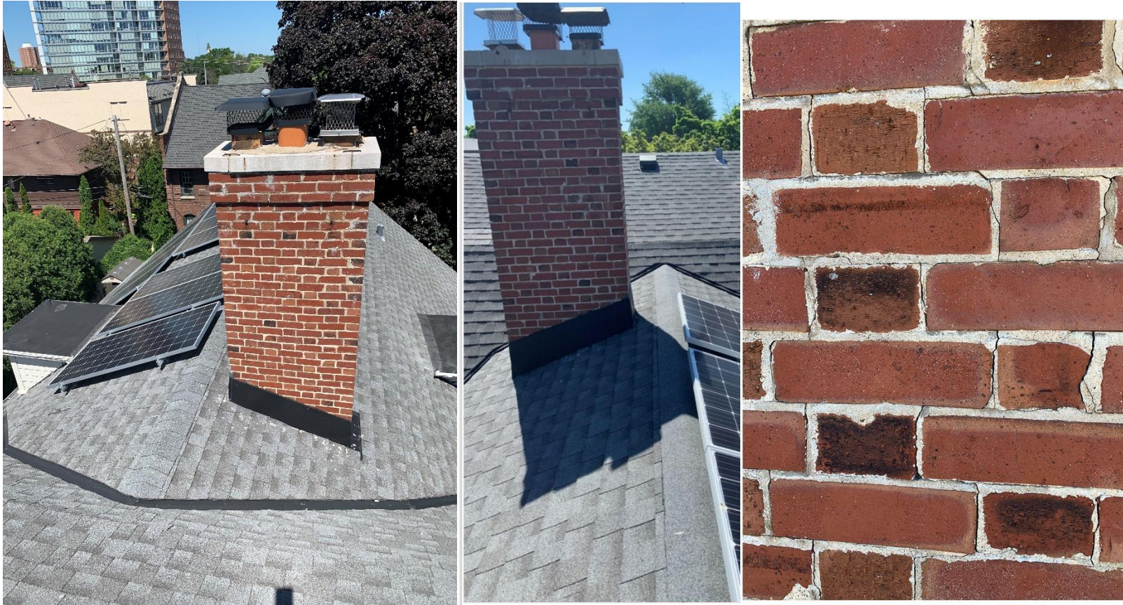
Abandoned chimney showing damaged areas
