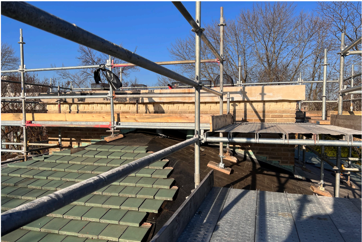
IMAGE 02: Photograph of scaffolding from flat roof to chimney cap. The existing roof tiles have been temporarily removed to gain safe access to the chimney and avoid damage to the tiles. These tiles are securely stored on-site and will be re-installed to match existing.
