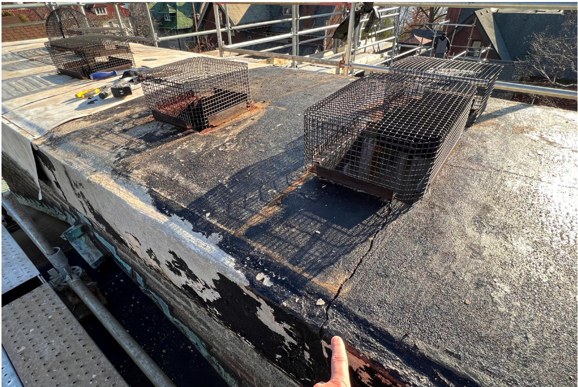
IMAGE 06: Photograph concrete chimney cap with rubberized asphalt adhesion/ waterproofing layer that exists beneath the roofing system. Hairline cracks in concrete cap observed at some re-entrant corners.
