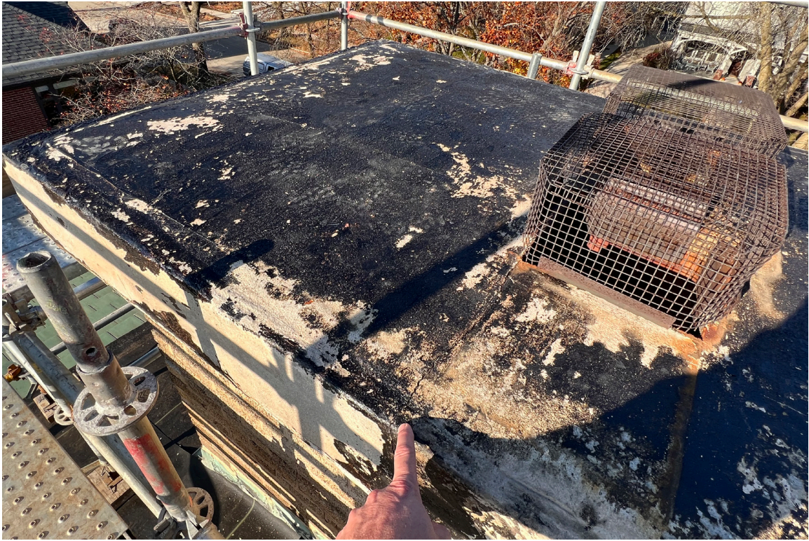
IMAGE 05: Photograph concrete chimney cap with rubberized asphalt adhesion/ waterproofing layer that exists beneath the roofing system. Hairline cracks in concrete cap observed at some re-entrant corners.
