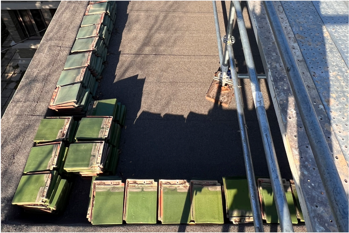
IMAGE 07: Photograph of existing roof tiles that have been temporarily removed to gain safe access to the chimney and avoid damage to the tiles. These tiles are securely stored on-site and will be re-installed to match existing.
