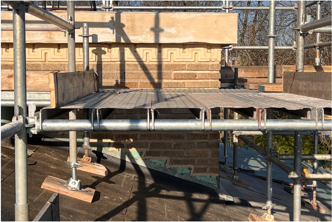
IMAGE 03: Photograph of stepped copper flashing at base of chimney and chimney cap with painted roofing system.
