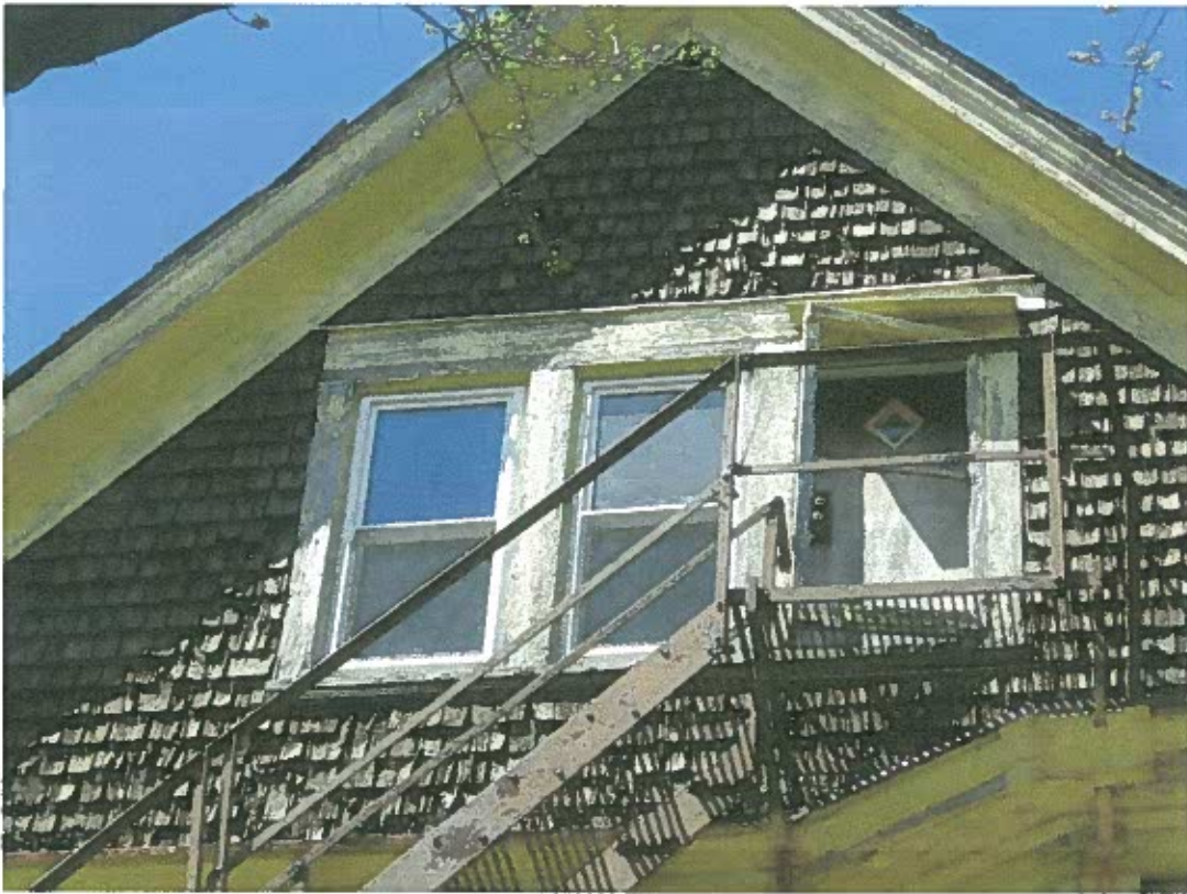
1. Wood Shingle Front Gable (East Elevation) attic window exit and fire escape stairs
