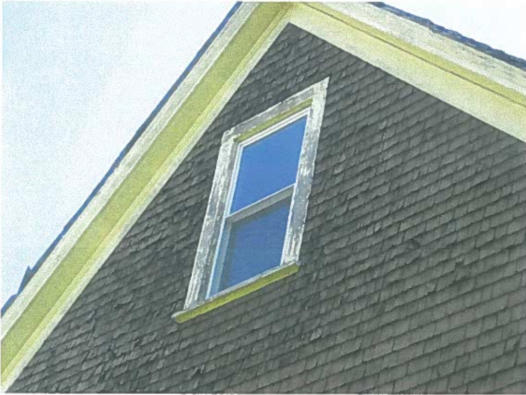
3. Wood shingle Rear Gable (West Elevation) showing shingle deterioration
