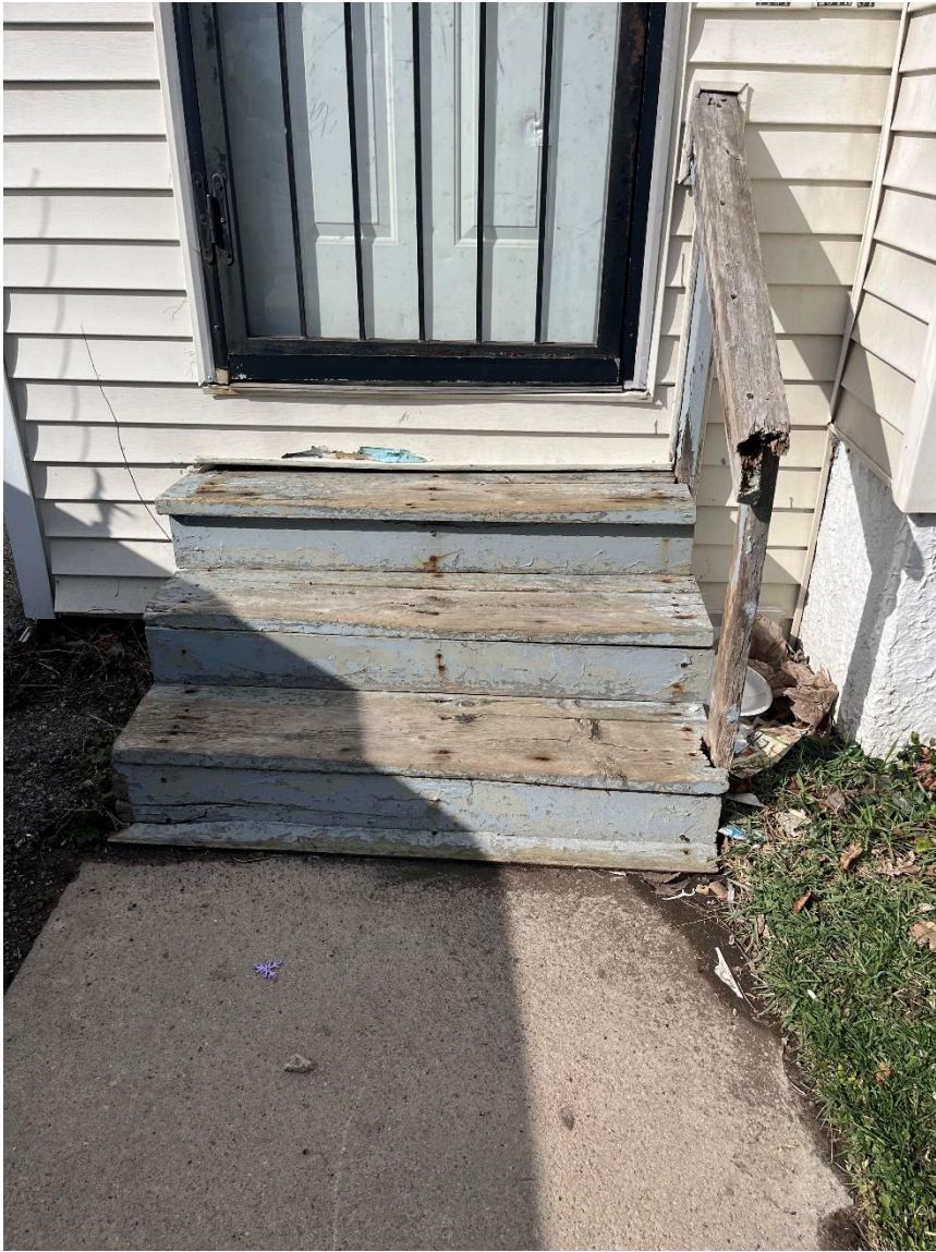
Stairs to be rebuilt.
