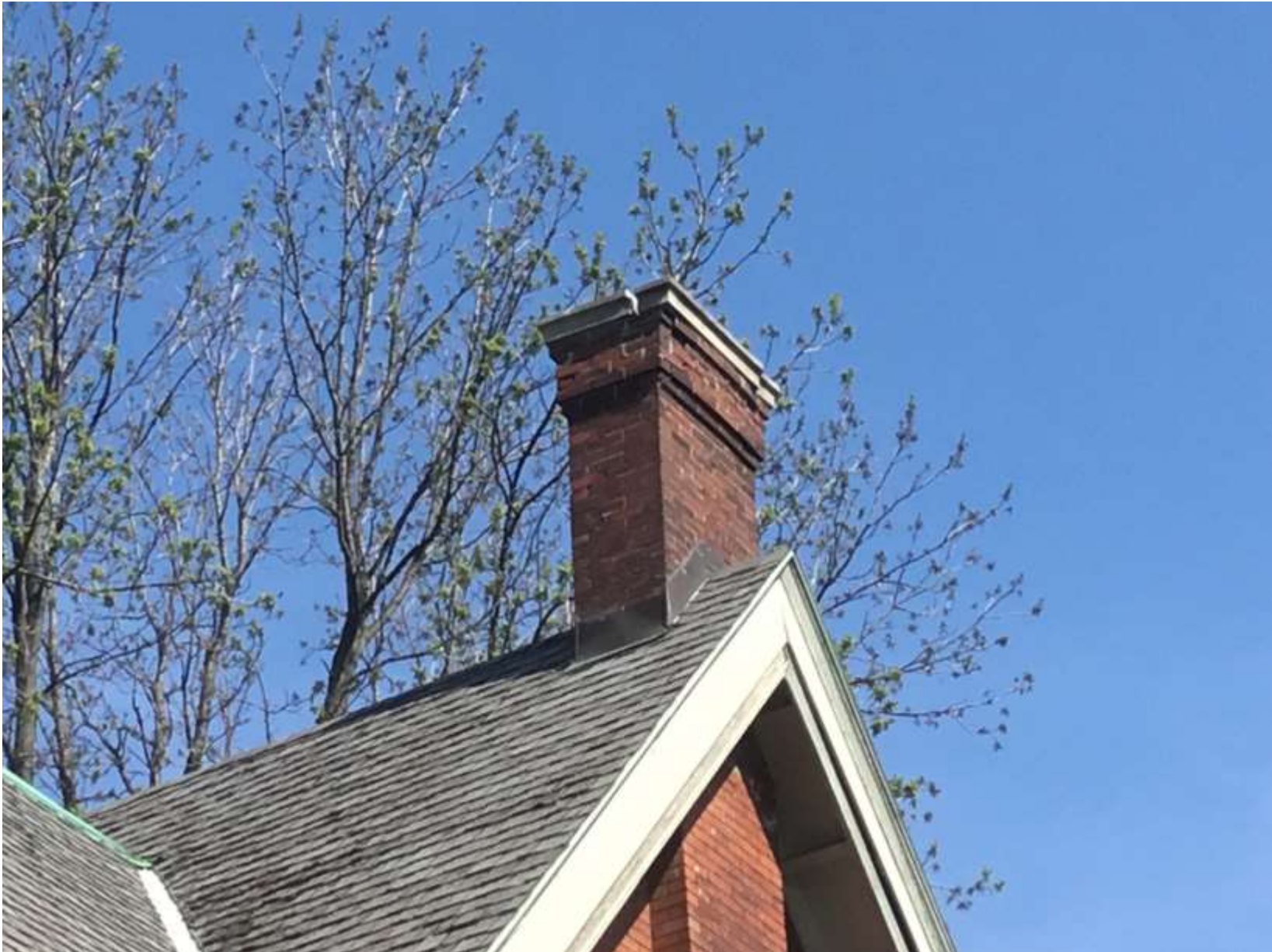
Detail of chimney. Existing flashing may remain, but cannot be re-installed in this manner if it is replaced. Corbelling details and stone/concrete cap must be retained.
