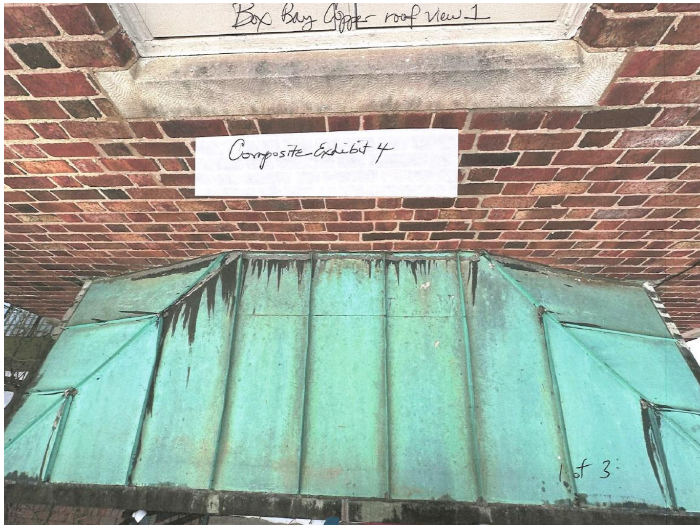
Replace in-kind the copper ribbed box bay window roof, copper flashing, and drip rail
