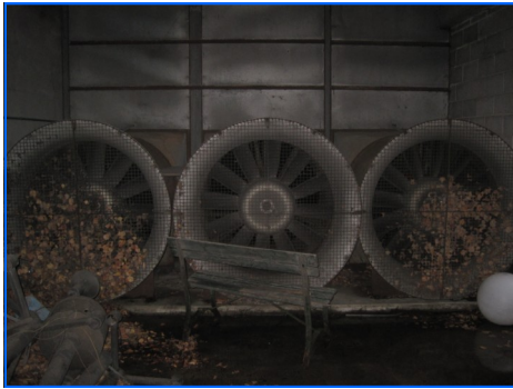
Typical exhaust fans
