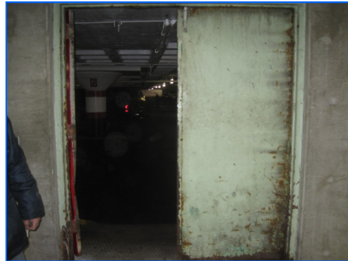
9th Street storage room door interior is rusted. Exterior is painted.
